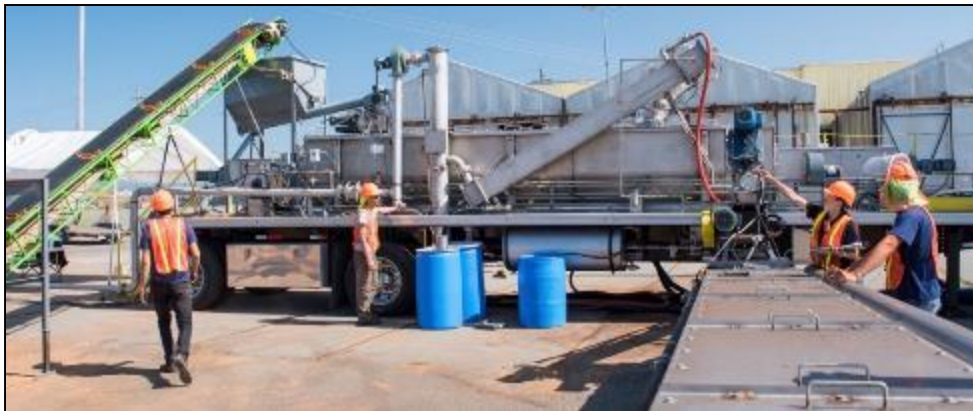
Torrefaction / Briquetting System
