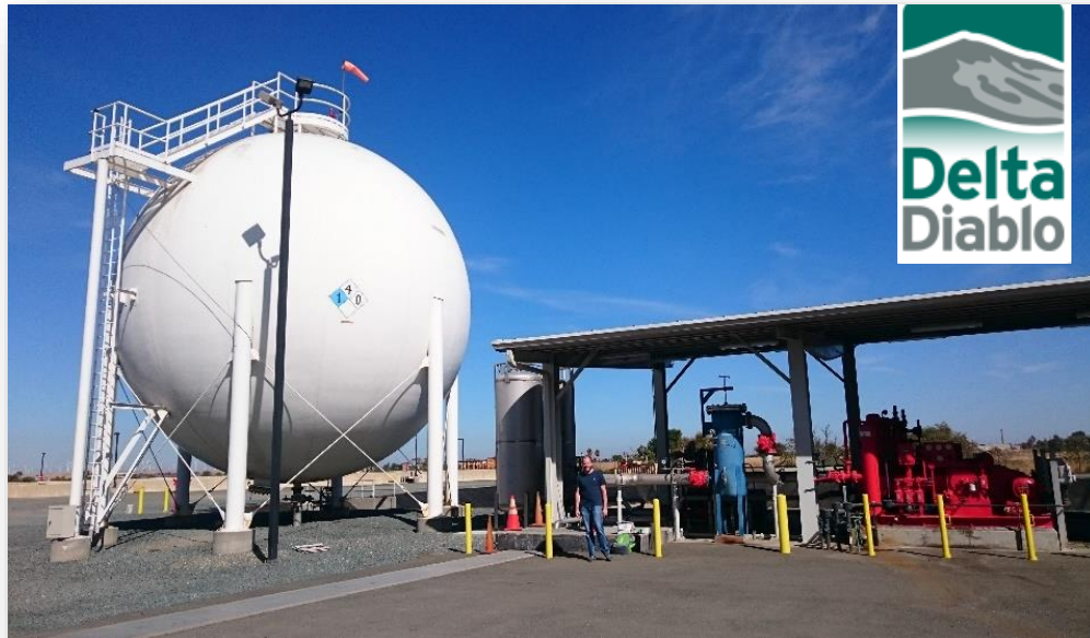
Sampling raw-biogas from Delta Diablo treatment plant.
