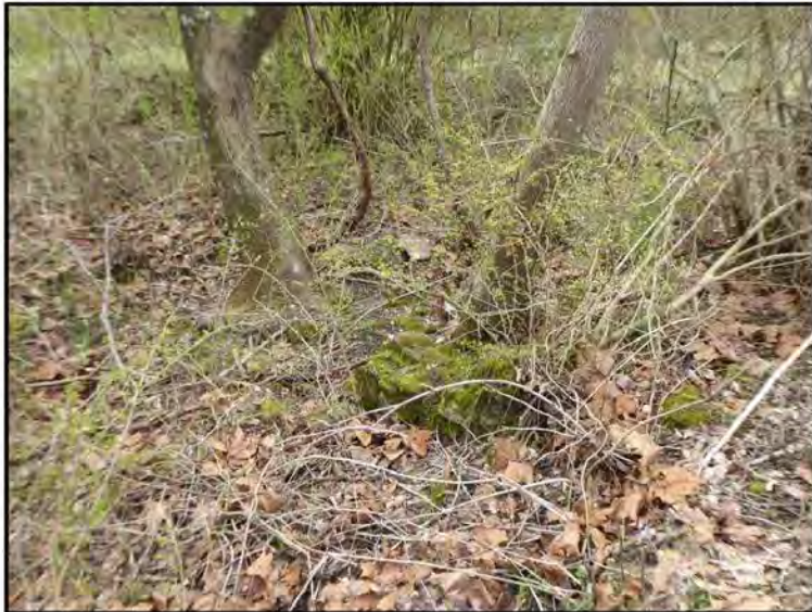
West foundation wall, facing south. Note interior portion of foundation in center of photograph.
