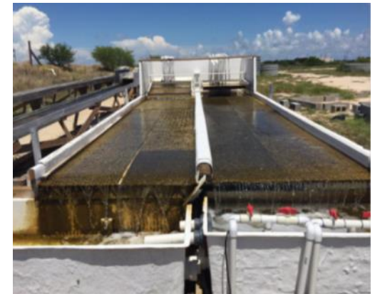
Algal Turf Scrubber at Corpus Christi, TX site
