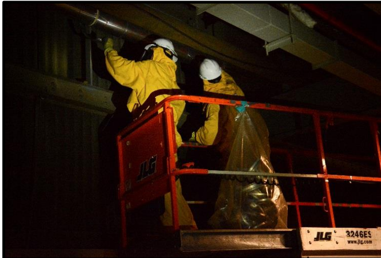
Using a scissor-lift, employees reach up to cut fiberglass insulation loose and pass it to workers below who bag it for disposal.
