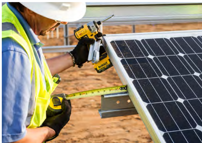
Solar Panels are installed at the 2-megawatt CoServ Solar Station in Krugerville, Texas.
