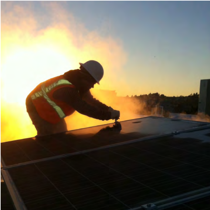
Solar installer installing a rooftop 36-kilowatt electrical PV installation for Reach Ashland Youth Center, a Leadership in Energy and Environmental Design (LEED) Platinum Certified building in Alameda County.
