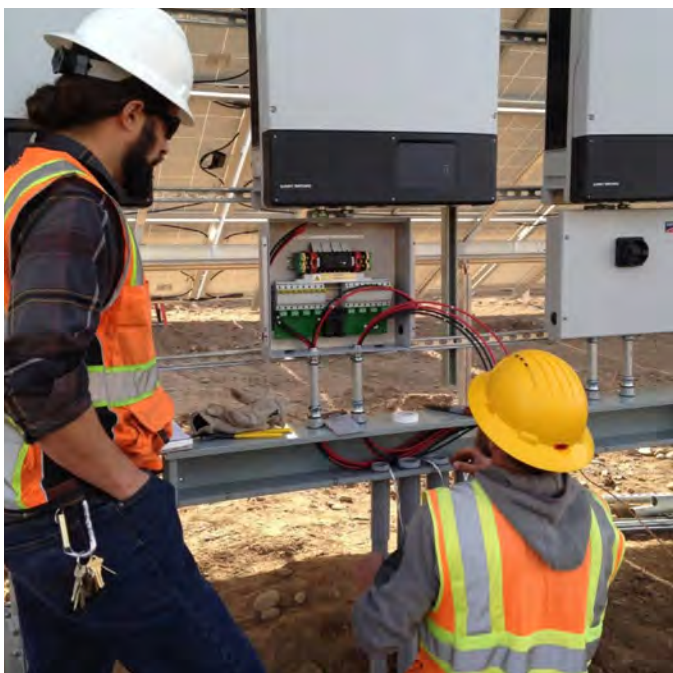
Sunsense solar technicians wire string inverters at the 234-kilowatt solar PV array powering the water treatment facility for the Town of Silt, Colorado.
