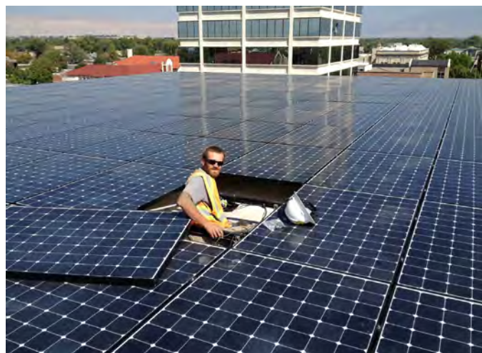
Final connections and troubleshooting are addressed on the 123-kilowatt solar electric system at the Wayne Aspinall Federal Building in Grand Junction, Colorado.
