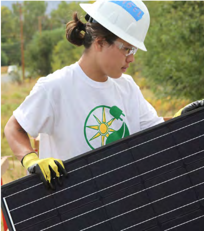
A GRID Alternatives volunteer helps with a solar installation on the Bishop Paiute reservation in California. Photo by Kate Costa.
