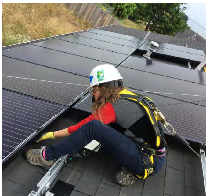
A GRID Alternatives volunteer helps install solar on a roof in Loleta, California.
