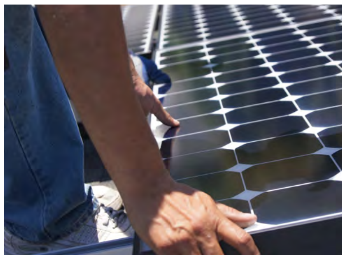
Solar installer lays a module on a California rooftop. Photo by Kate Costa.
