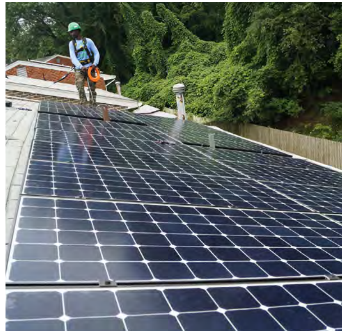
Solar installer laying out conduit after solar panels have been installed on a home.
