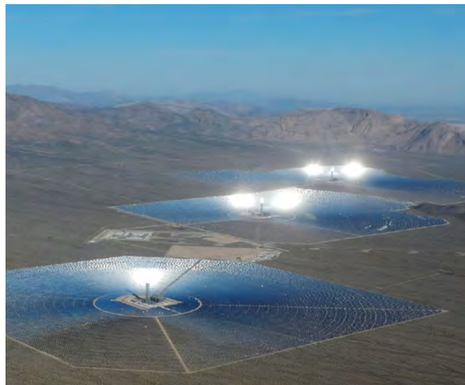
Aerial photo of Ivanpah Solar Electric Generating System taken from a helicopter on March 23, 2015. Photo by Cliff Ho.
