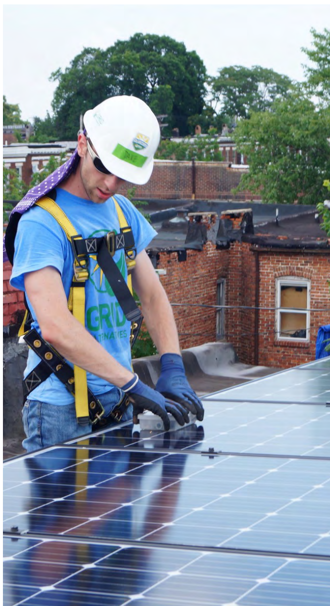
Dave, a solar installation supervisor working at GRID Alternatives Mid-Atlantic, inspects the solar panels after installing for a low-income family in Baltimore, Maryland.
