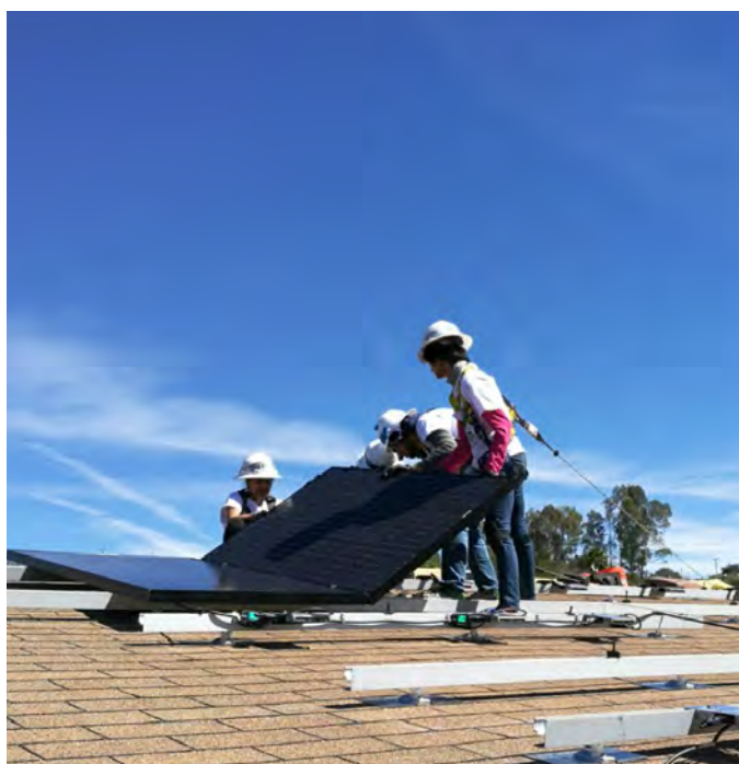
GRID Alternatives' volunteers, Jigeesha Upadhyaya and Raginee Yadav, from Arizona State University's professional science master's program installing a 5-kilowatt rooftop system in San Pasqual, California.
