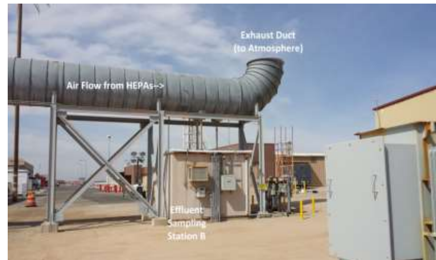
Effluent Sampling Station B
