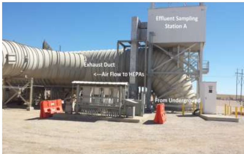
Effluent Sampling Station A
