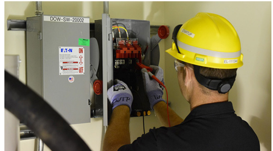
Photo 1. An electrician tests control panel switches in Hanford's Analytical Laboratory.
