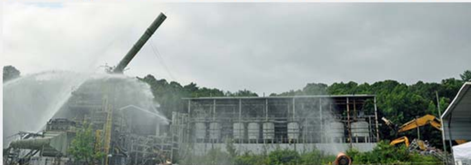
Crews take down a 100-foot stack at the Toxic Substances Control Act Incinerator.
