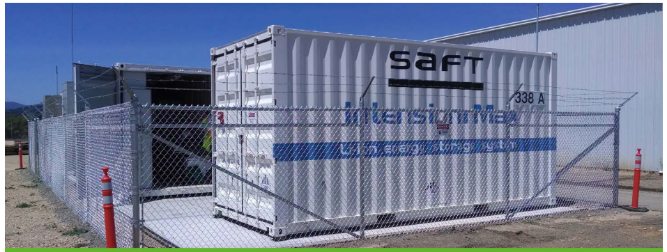
Figure 1. Fort Hunter Liggett installed a lithium-ion battery to help mitigate demand charges and reduce PV curtailment. The battery was purchased with funding from the Army's Energy Resilience & Conservation Investment Program. Photo by Lars Lisell, NREL.
