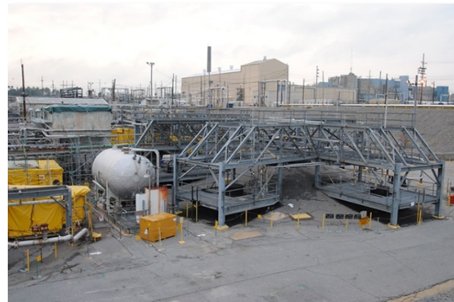
Tank 20 at the Savannah River Site
