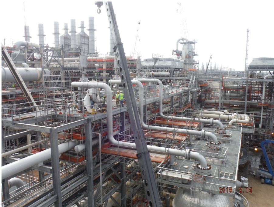
Train 5 – Dehydration Mercury Removal Area
