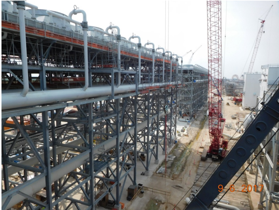
Train 5 - Propane Condenser Rack
