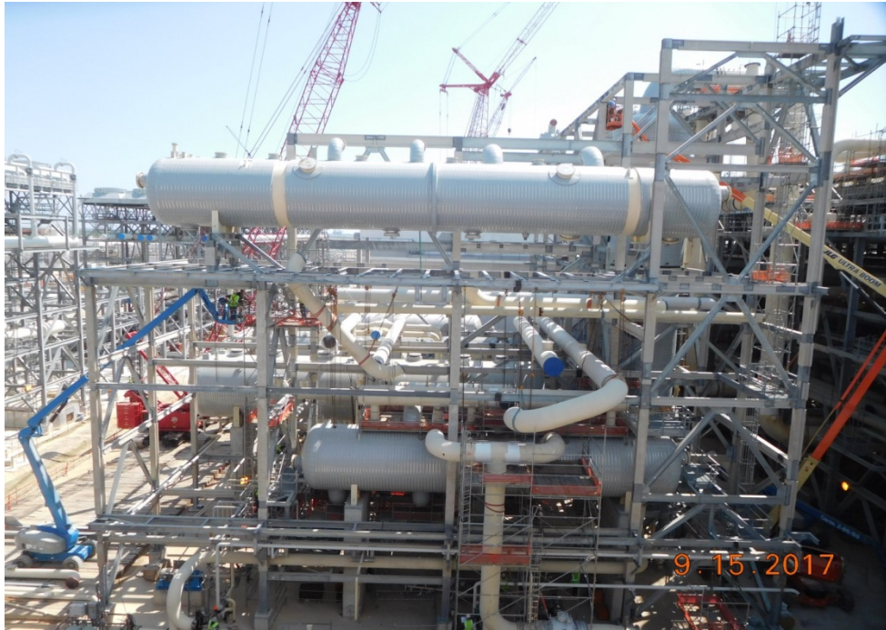
Train 5 – Propane Refrigeration Area
