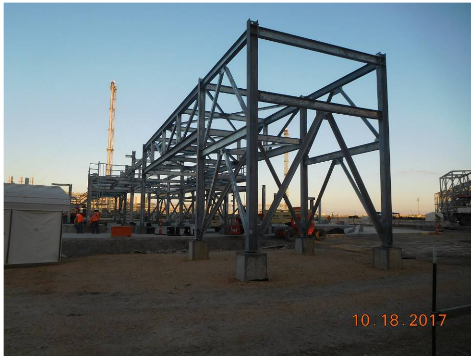
Stage 3 OSBL – Elevated Flare Rack (Flare Modification Scope)
