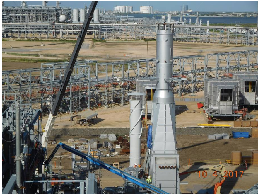
Train 5 –Thermal Oxidizer (Flare Pipe Rack in OSBL in the background)
