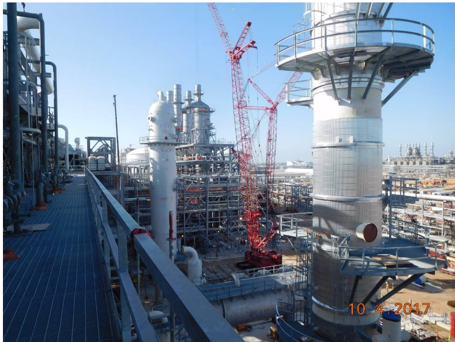
Train 5 - West side of ISBL viewed from the top of AGRU Rack
