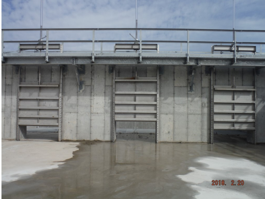
OSBL – Outfall Inlet Sluice Gates
