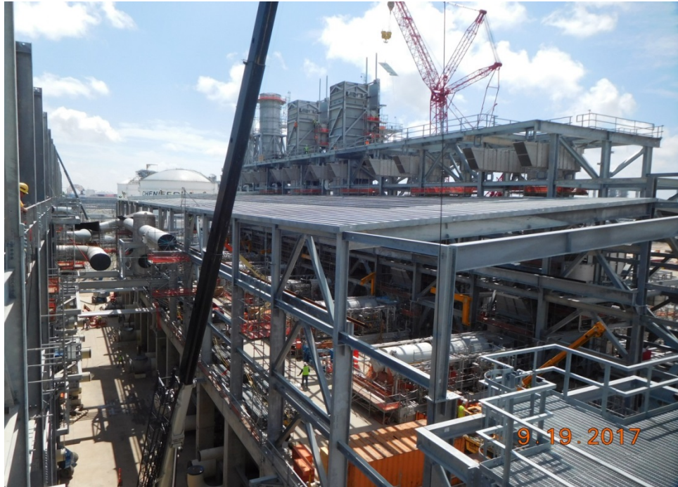
Train 5 - Compressor Area
