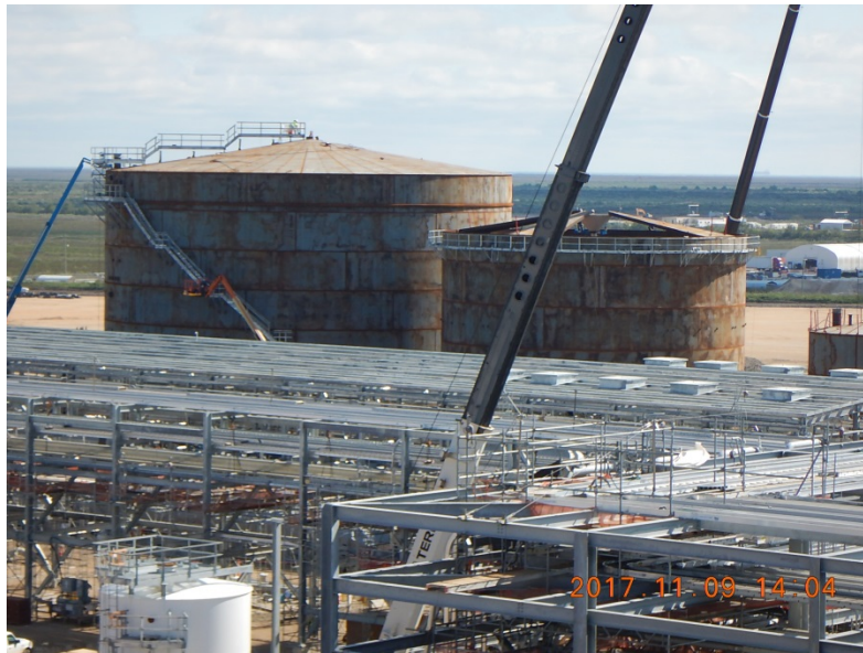
OSBL – Field Fabricated Tanks
