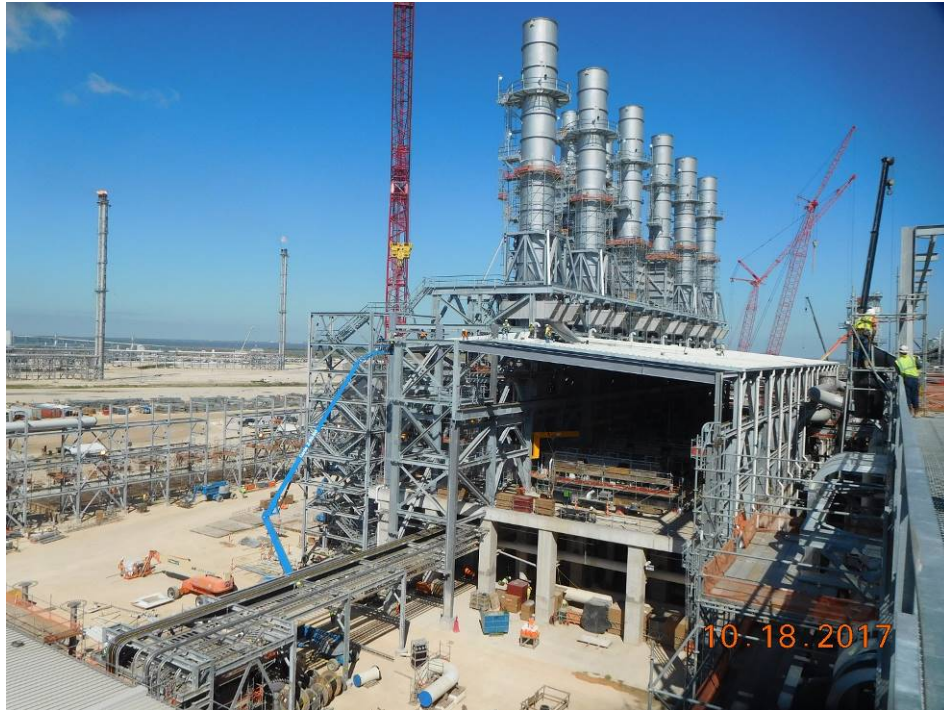
Train 5 – Compressor Area
