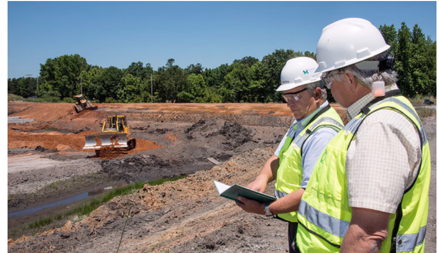
Picture 3. Work with heavy equipment presents hazards to the operator and bystanders. Pictured here, Savannah River Nuclear Solutions environmental engineers inspect plans for earth-moving work within a basin containing coal ash.
