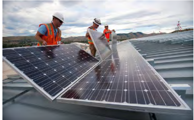
Roof-mounted solar panels help the Research Support Facility reduce its carbon footprint.
