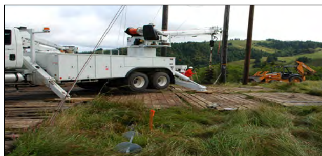
BPA installs temporary wood mats over wetlands to minimize impacts from heavy vehicles and equipment during construction of transmission line structures.
