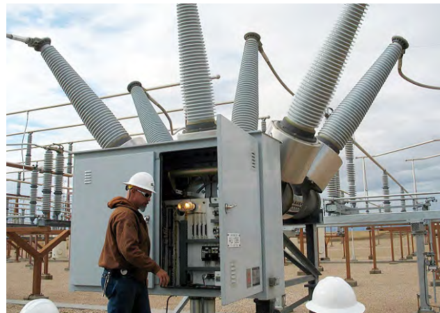
A Western Area Power Administration electrician checks a circuit breaker, which contains 85 pounds of sulfur hexafluoride to protect substation equipment from excessive electrical currents.
