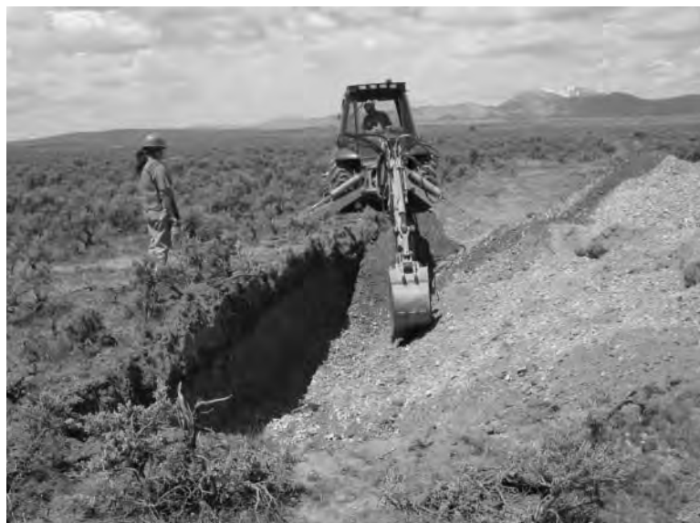
A tribal representative monitors trenching operations for cultural resources at a site near the Big Lost River.
