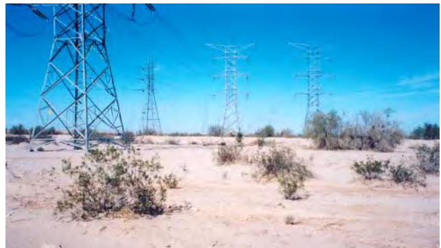
Electric transmission lines extend north from Mexico across the international border (which is the berm across the center of photo). Inside the U.S., the lines are constructed on BLM land.
