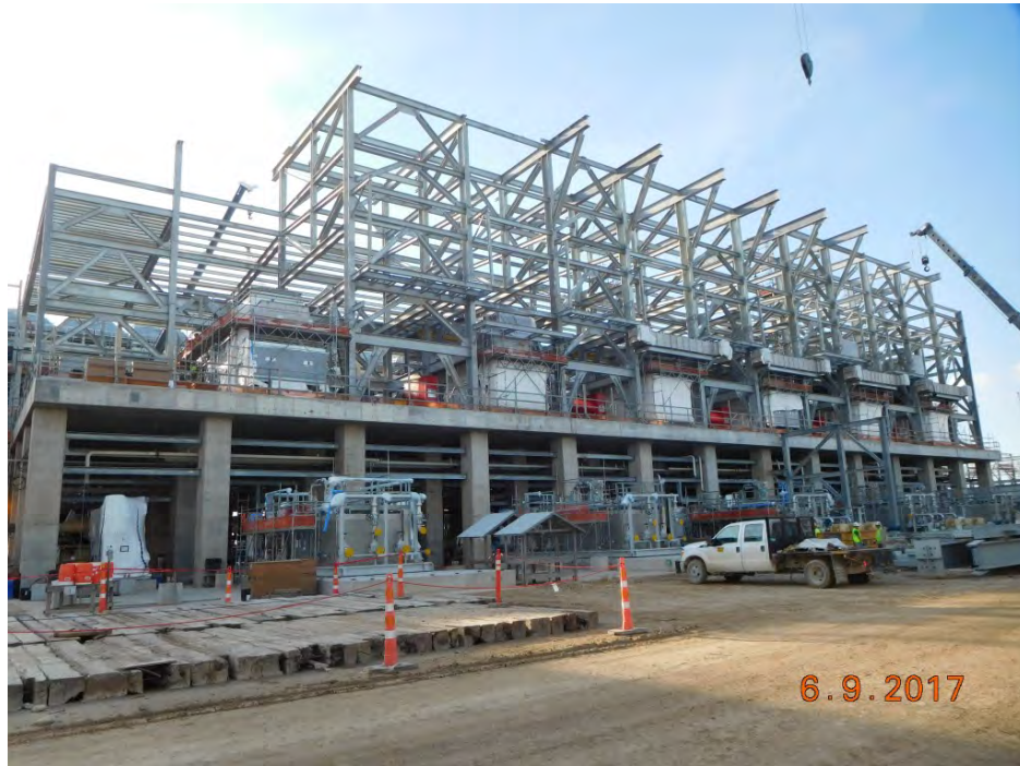
Train 5 – Compressor Area
