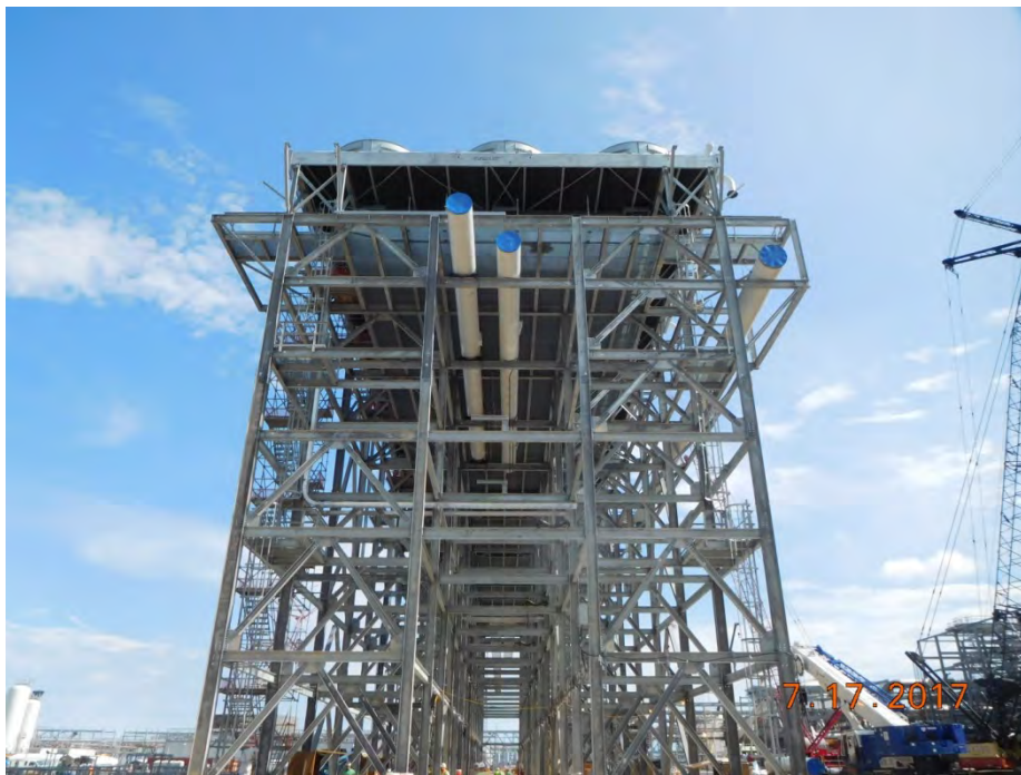
Train 5 – First Large Bore Pipe in South Side of Propane Condenser Rack
