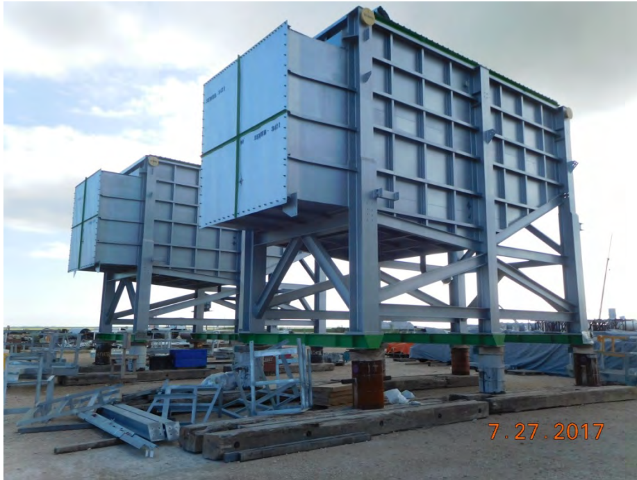
Train 5 – Waste Heat Recovery Unit (Bottom Part) in Laydown
