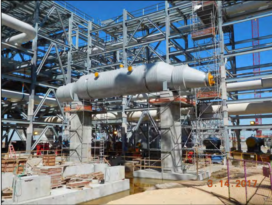
Train 5 – H.S. Propane Feed Chiller In Hydration Area
