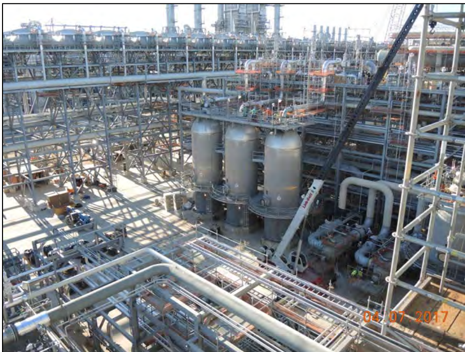
Train 4 – View From Top of Cryo Rack
