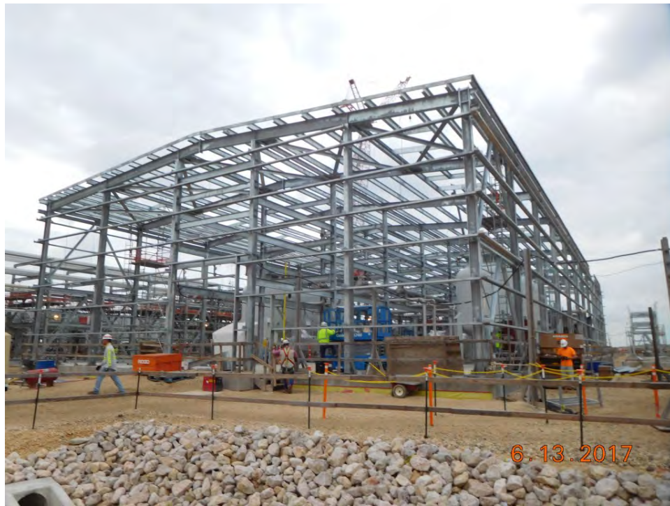
Stage 3 OSBL – Water Treatment Area
