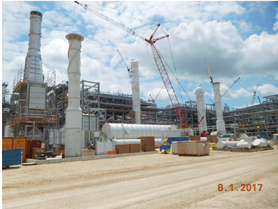
Train 5 – Thermal Oxidizer Area
