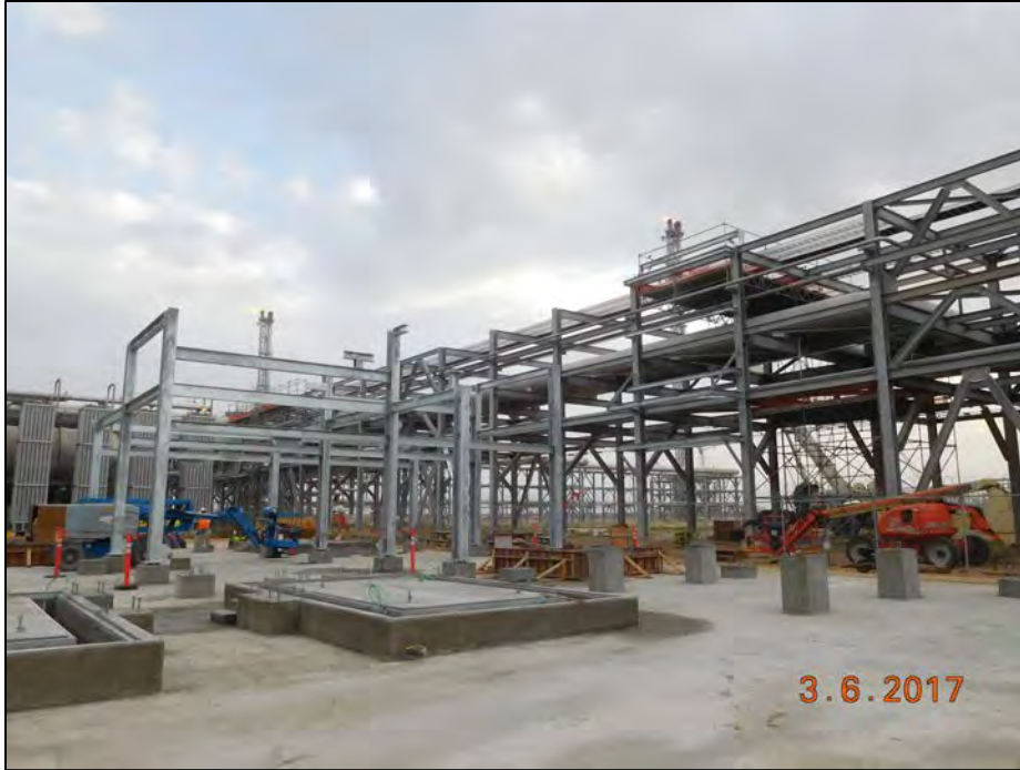
Stage 2 – HPA Flare Compressor Area
