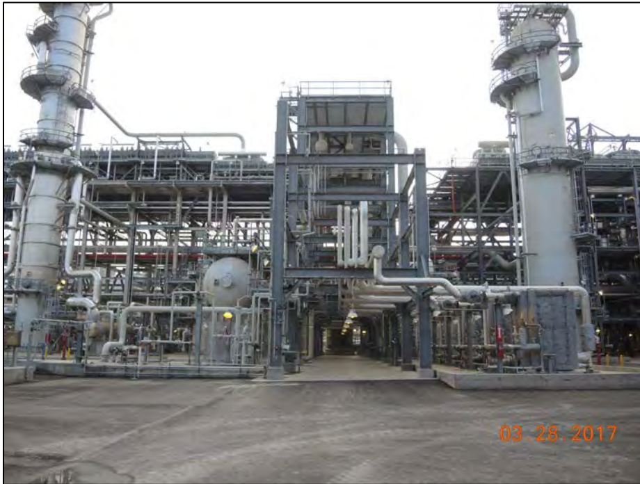
Train 3 – Amine & Acid Gas Removal Area
