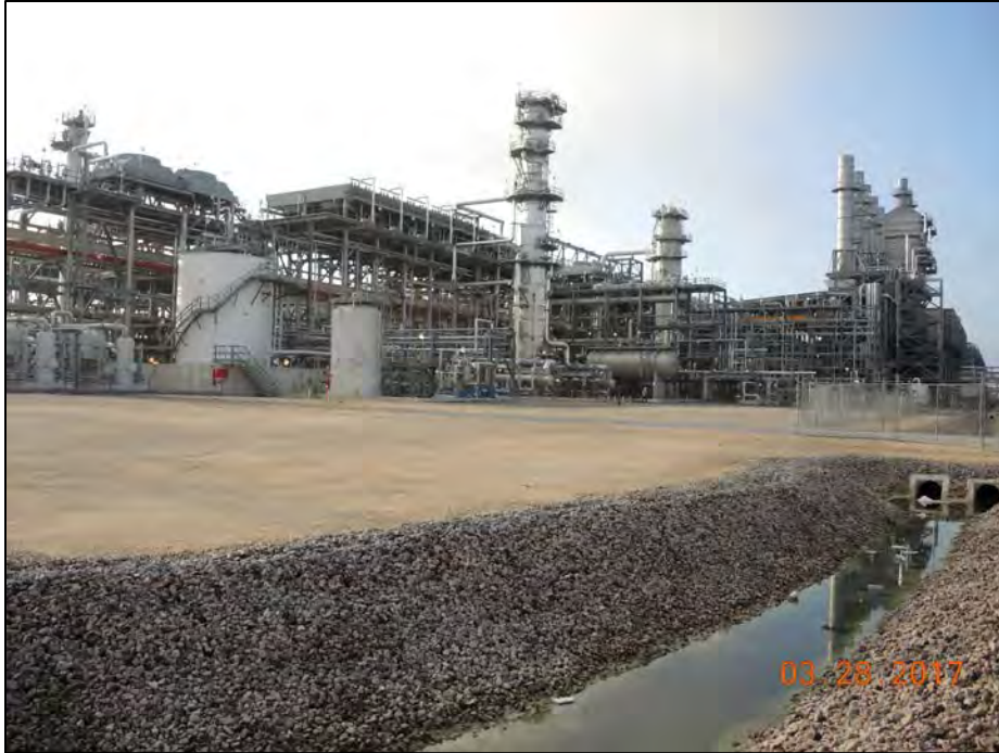
Train 3 – View From The Northwest Corner of ISBL
