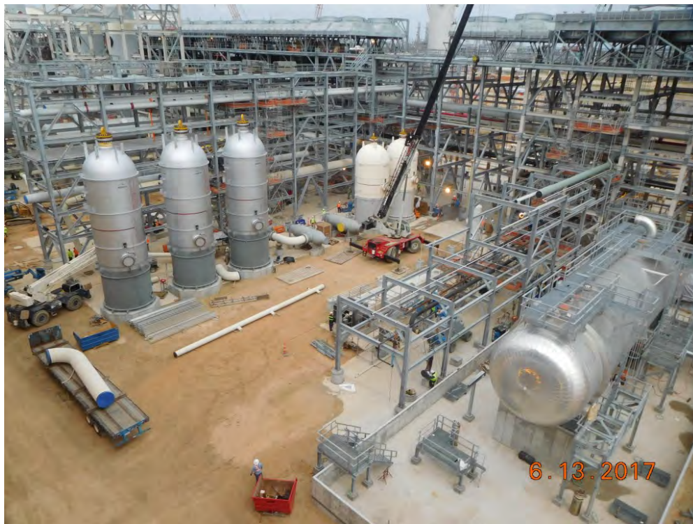
Train 5 – Dehydration / Mercury Removal and Hot Oil Areas
