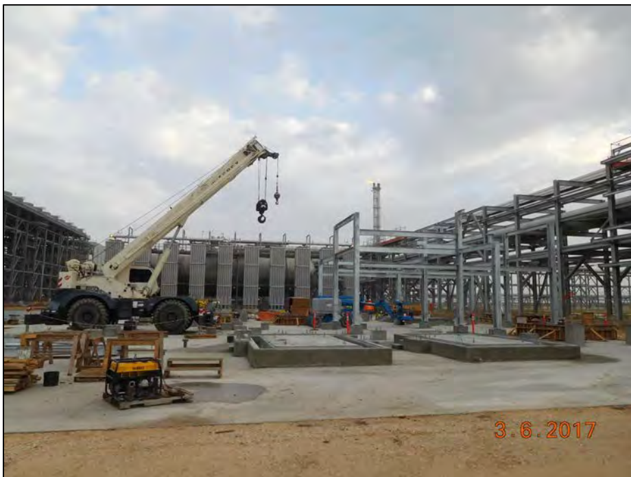
Stage 2 – HPA Flare Compressor Area
