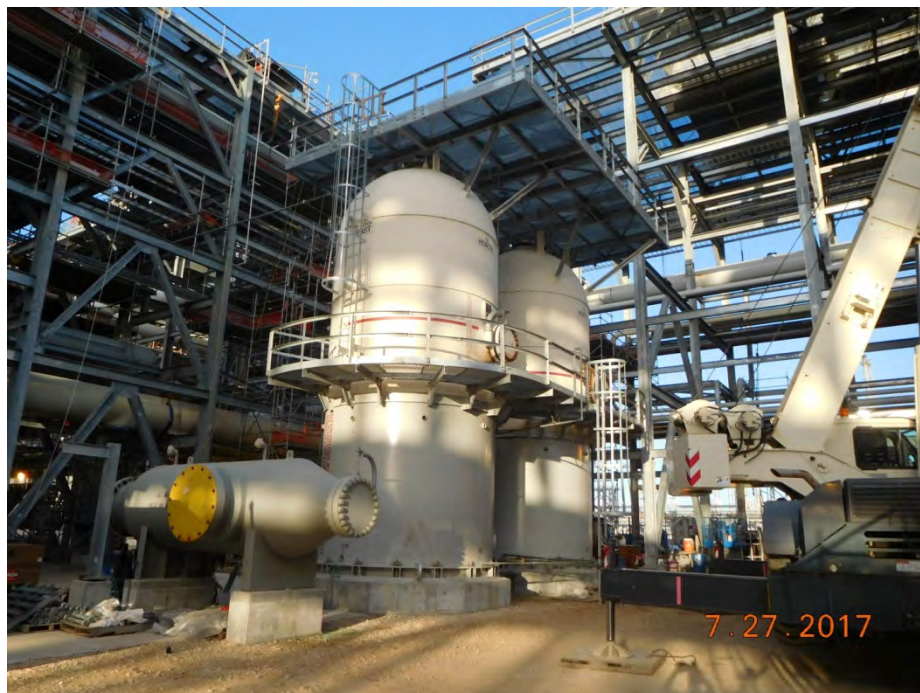
Train 5 – Mercury Removal Beds (1304A-B) in Mercury Removal Area
