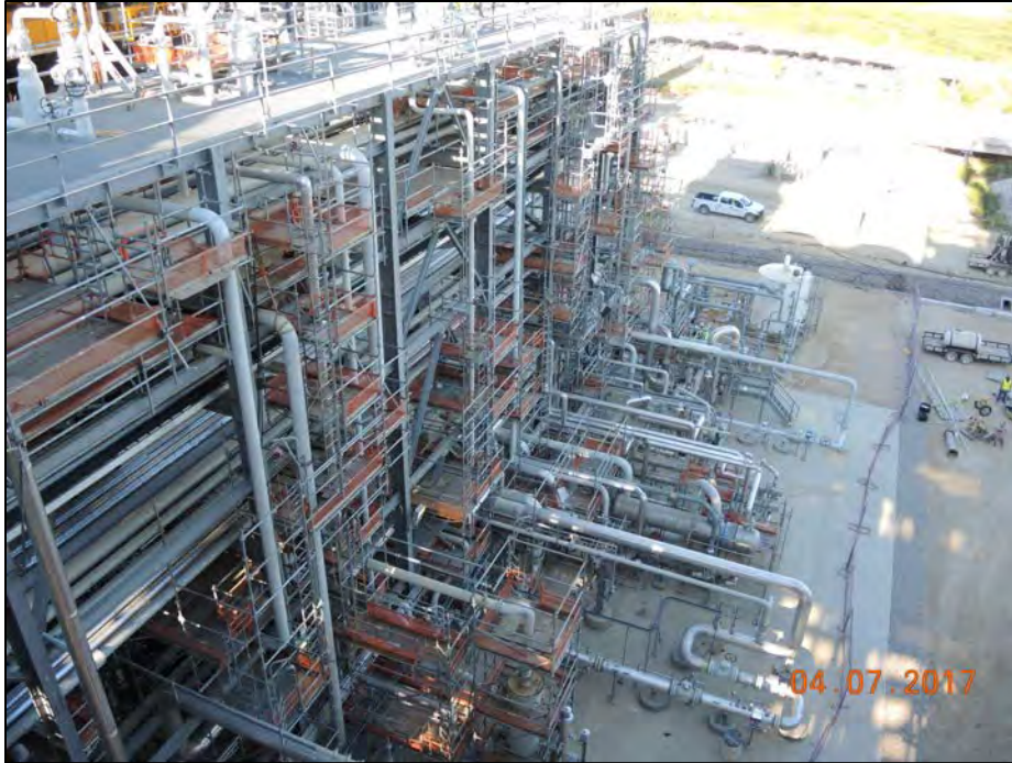
Train 4 –Fuel Gas Area
