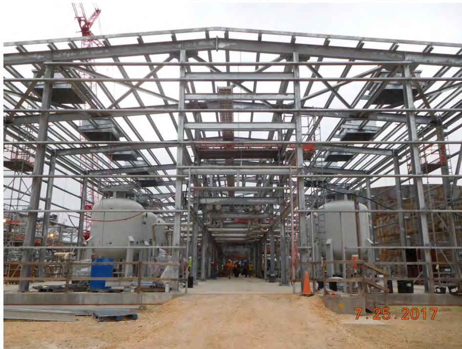
Stage 3 OSBL – Water Treatment Area
