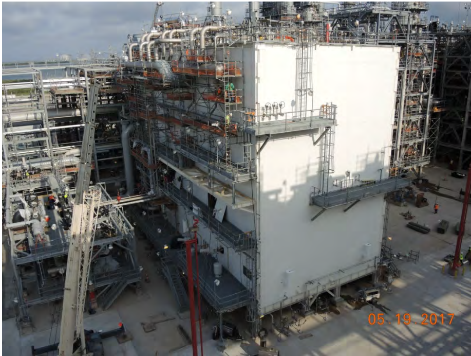
Train 4 – Methane Cold box
