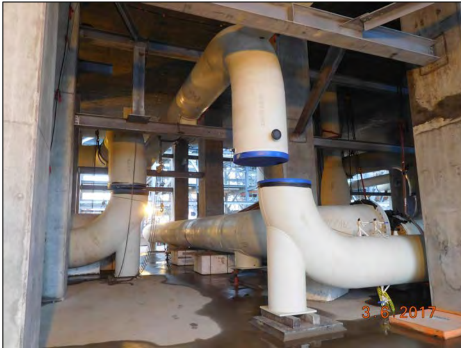
Train 5– Large Bore Piping Under Compressor Deck
