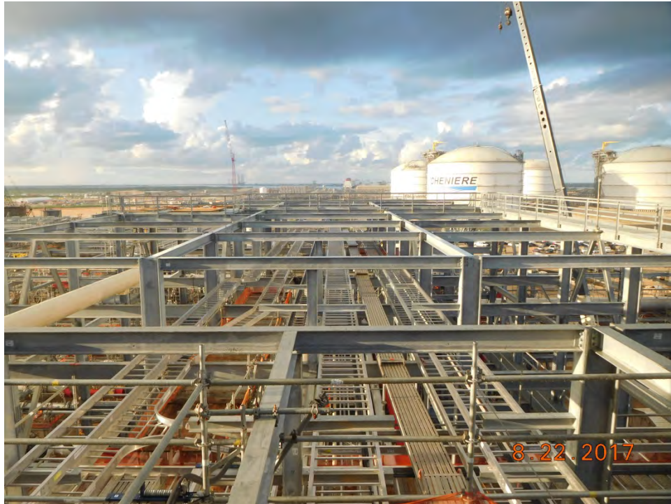
Train 5 - South Side of Cryo Rack (Upper Level Steel)
