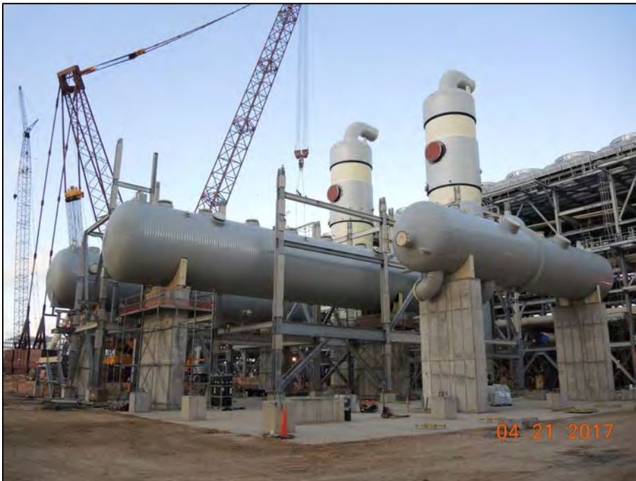
Train 5 – Propane Refrigeration Area
