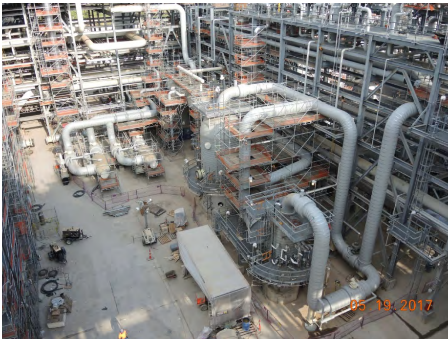
Train 4 – Mercury Removal & Dehydration Area – North
