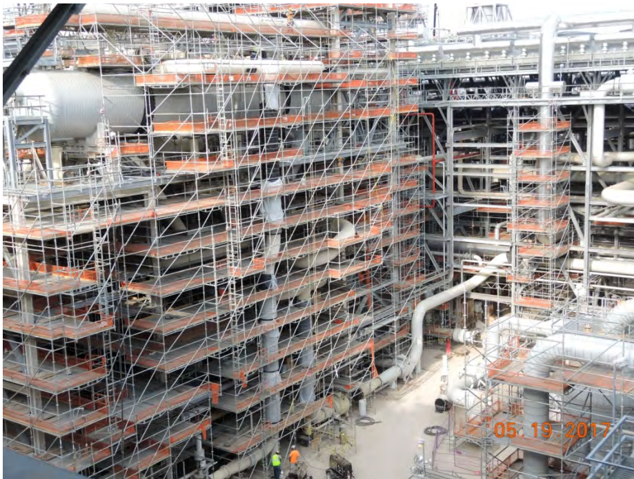
Train 4 – Propane Refrigeration Area
