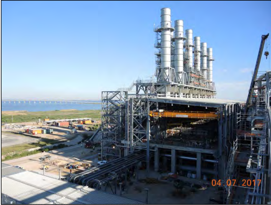
Train 4 – Compressor Area
