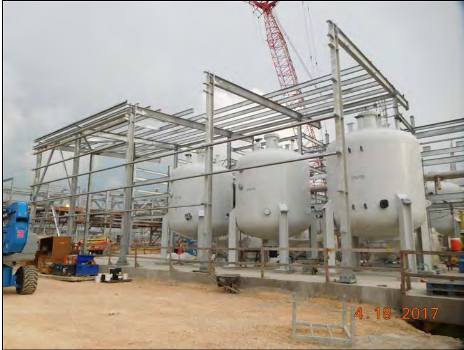
Stage 3 OSBL – Water Treatment Building
