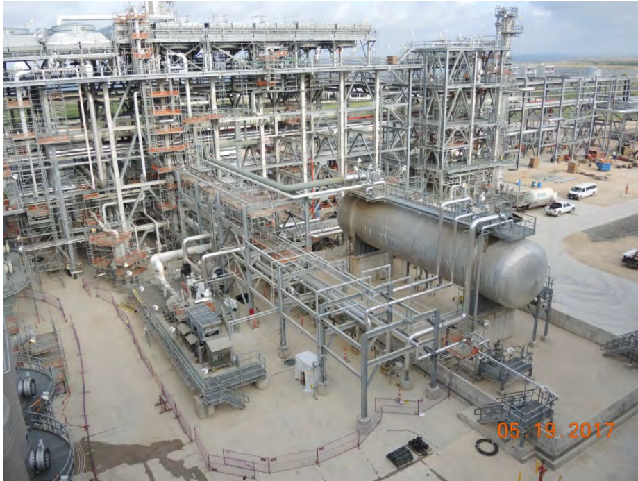
Train 4 – Hot Oil Area
