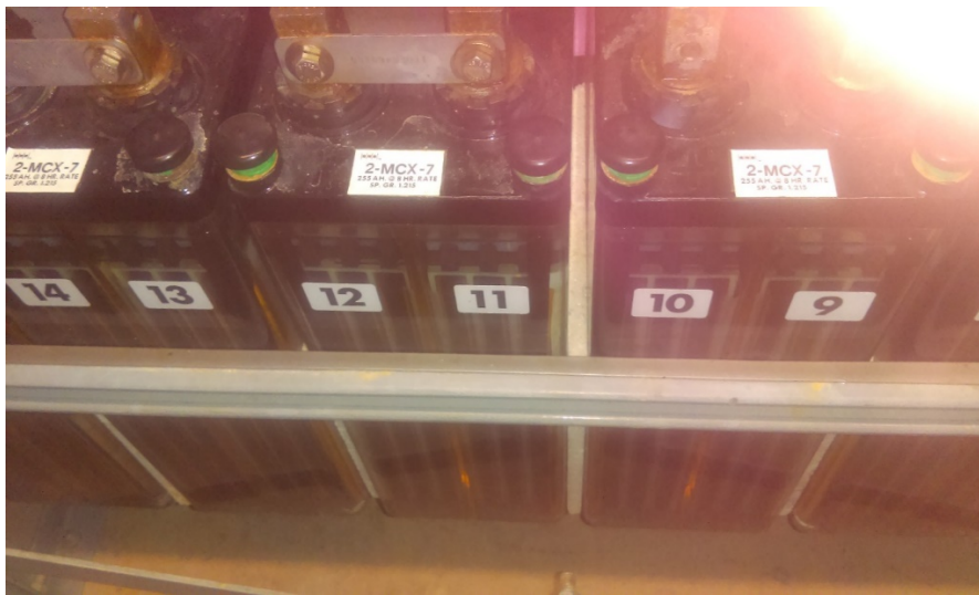
Figure 1. Failed Battery Cells 9/10
