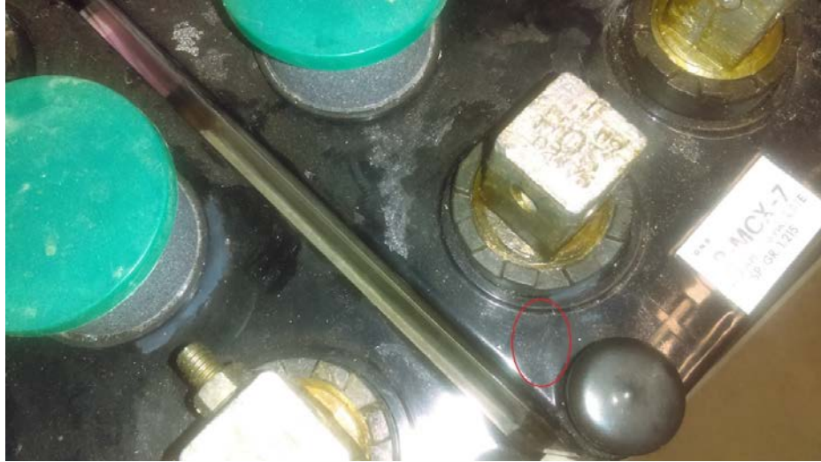
Figure 2. Cover of Cell 10 Highlighted in Red Oval where crack occurred
