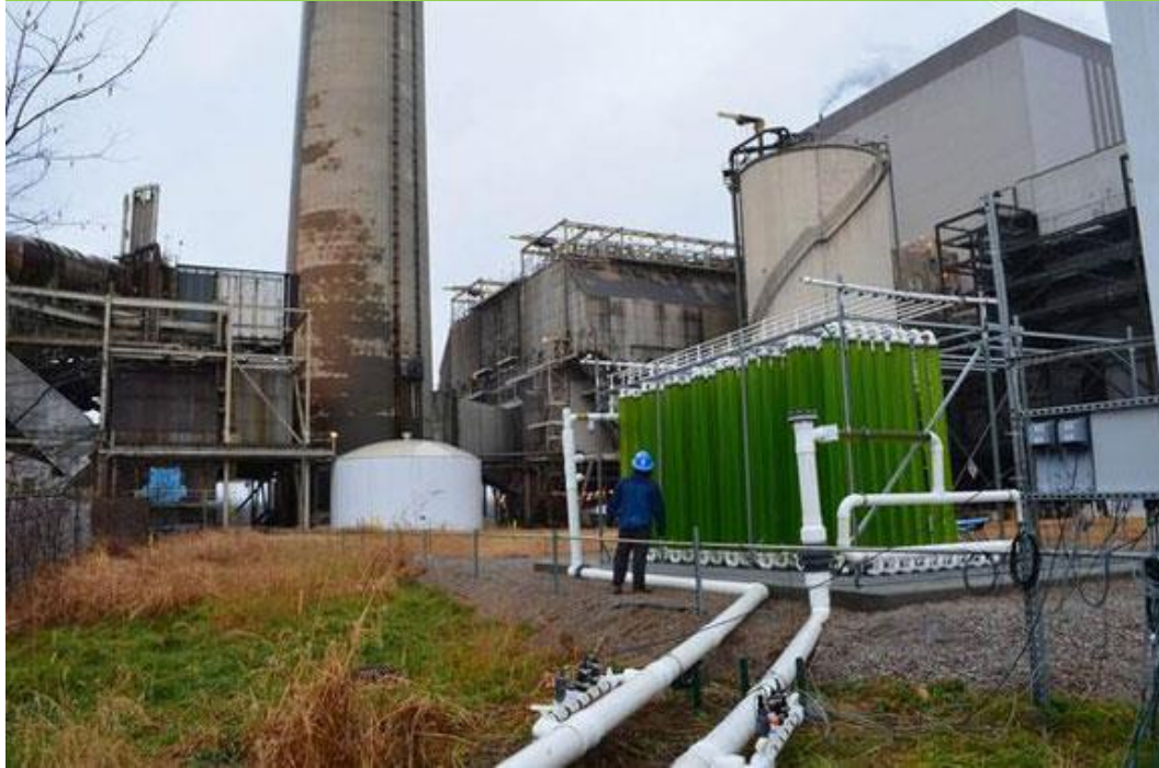
U of Kentucky – Duke Energy’s East Bend Station
