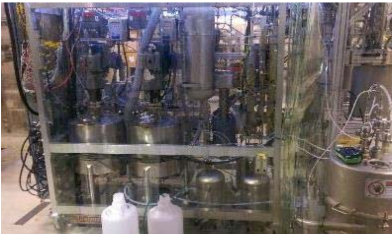
Slurry Feed system
