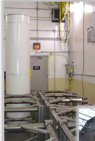
TWPC Canister Storage Room
