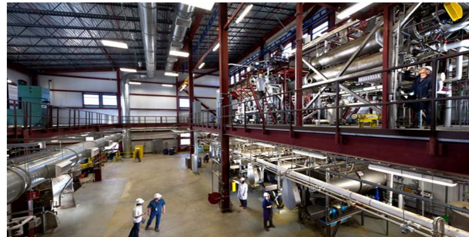
NREL's Integrated BioRefinery Research Facility (Pilot Scale)
