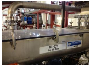
Inefficient online acid mixing
