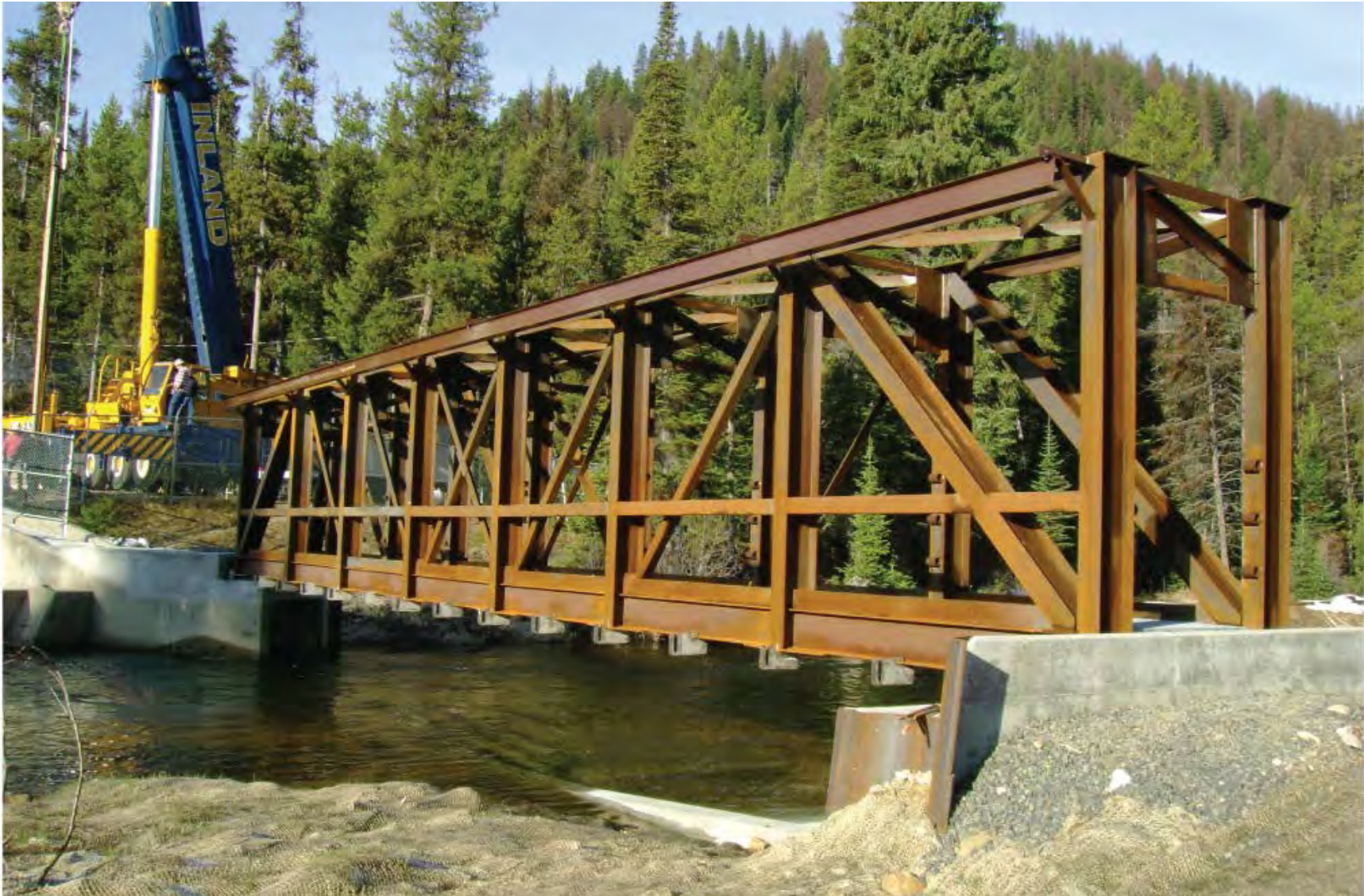
Figure 2-6a. Example of Bridge Weir Fully Constructed (South Fork Salmon River Bridge Weir)
