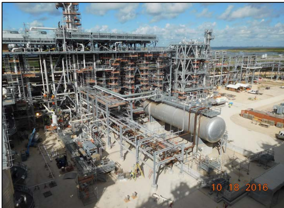
Train 4 - Hot Oil Area
