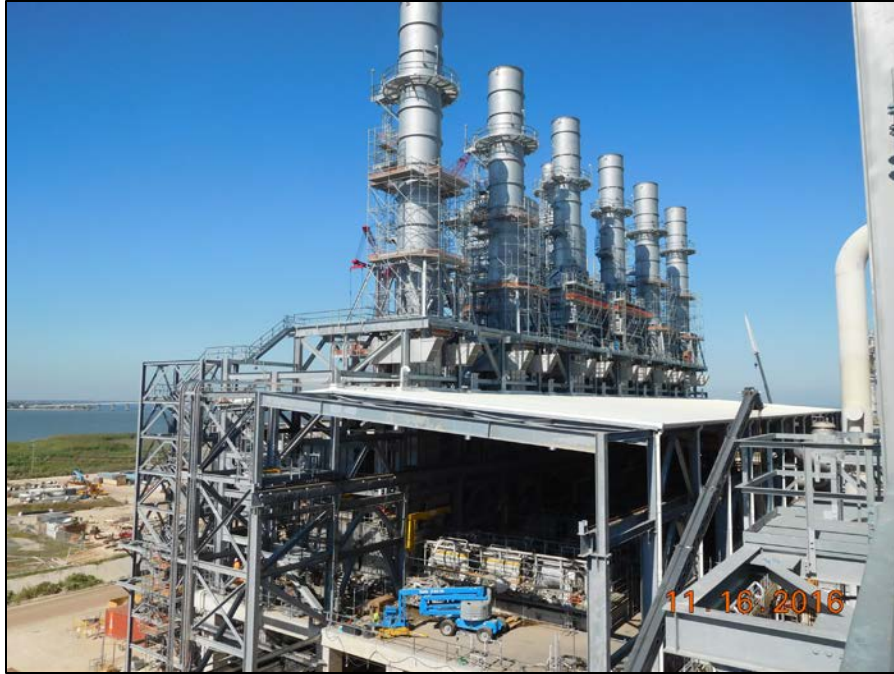
Train 4 - Compressor Area
