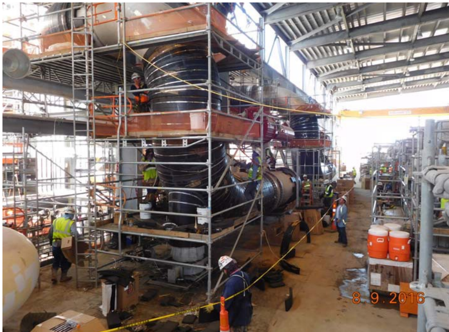
Train 3 - Insulating Pipe Above the Compressor Deck
