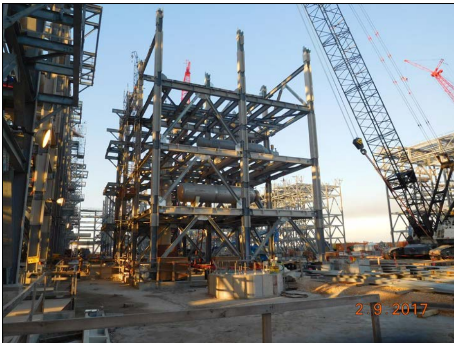
Train 5 – M01 Structure and Equipment
