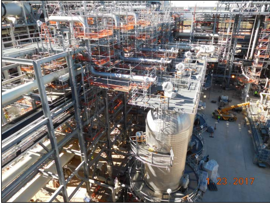
Train 4 – Hydraulic / Mercury Removal Area
