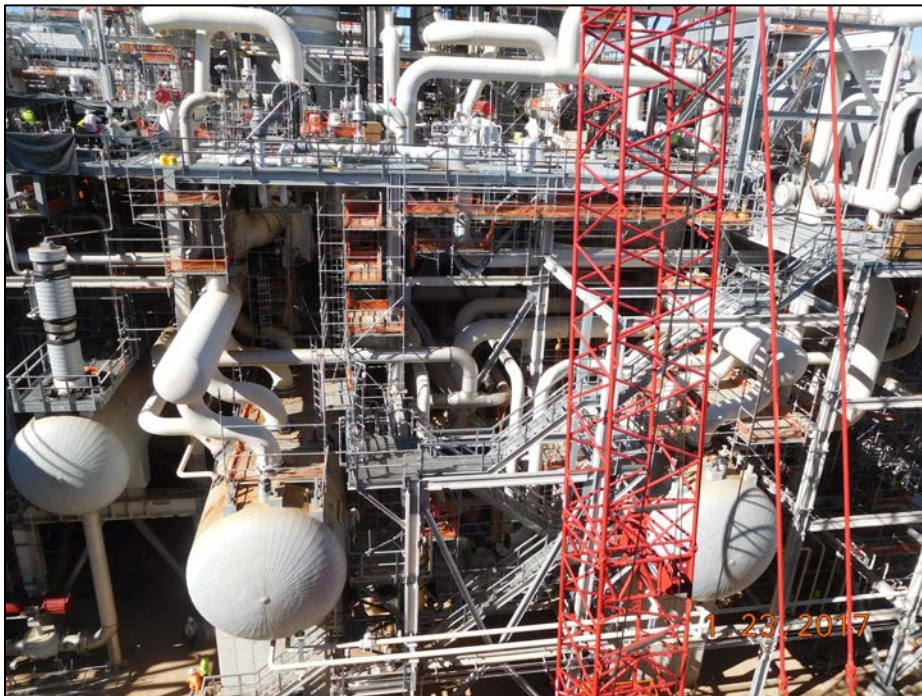
Train 4 – Propane Refrigeration Area
