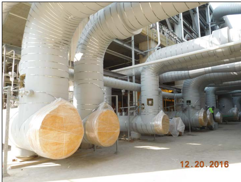
Train 3 - Pipe Insulation in Alleyway Between Compressor Deck & Cryo Rack
