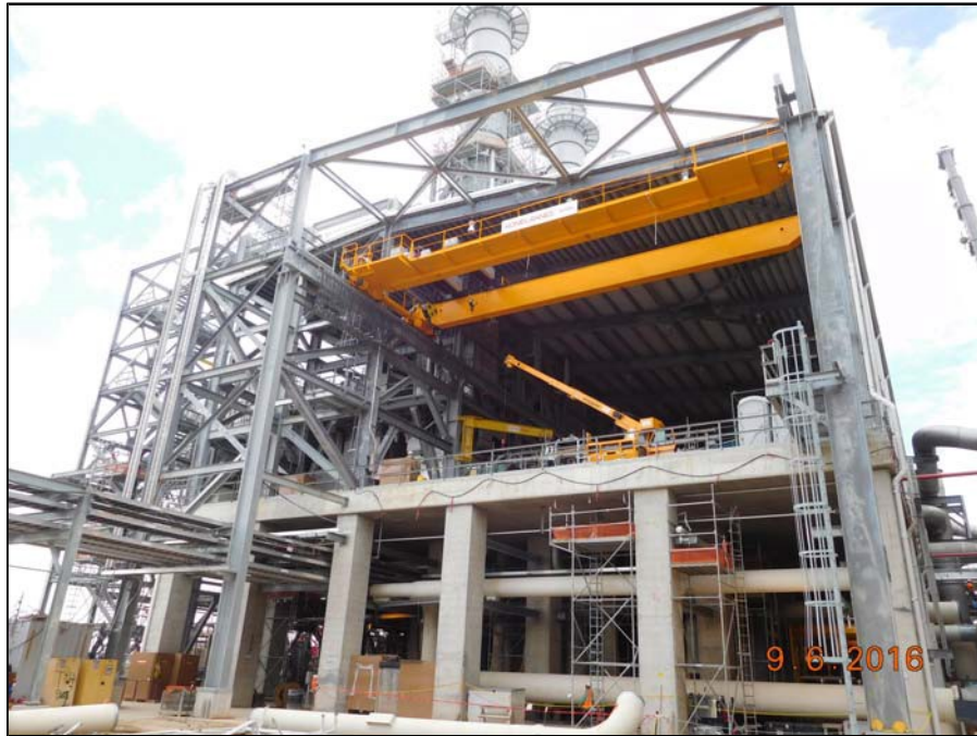
Train 4 - Compressor Area Bridge Crane
