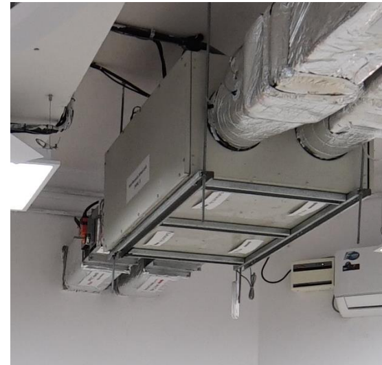
Heat recovery wheel
