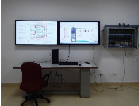
Control room for the FDD test facility at IIIT Hyderabad
