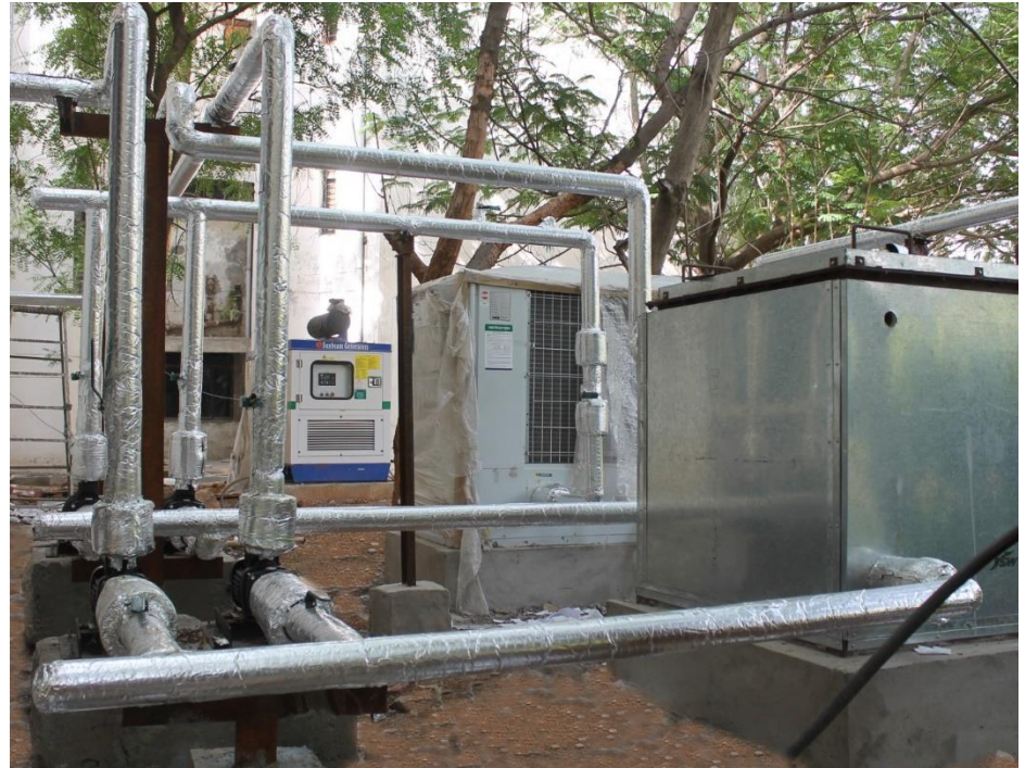
Dedicated chilled water plant for the FDD test facility at IIIT Hyderabad
