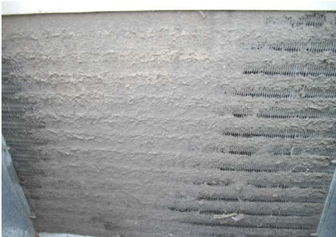
Fouling of evaporator coil 3
