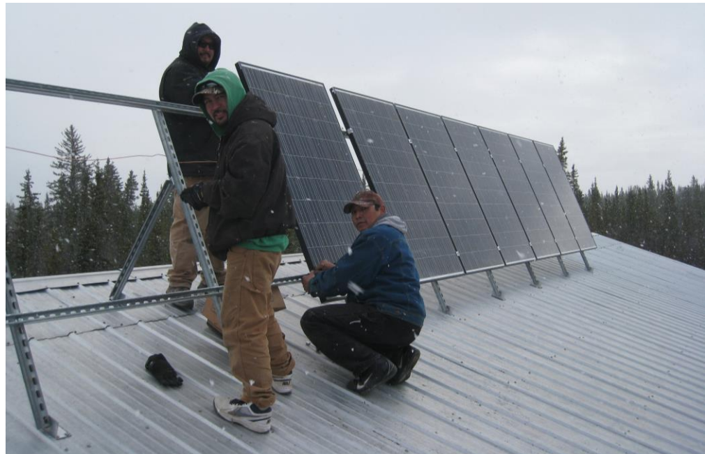
Figure 1. Gwichyaa Zhee Gwich'in Tribal government Employees working on the construction of the Fort Yukon 18kW Solar PV array on the Fort Yukon Tribal Hall in May of 2015. from top left down and to the right Jacob wright, Clayton Tackett and Gerald Alexander
