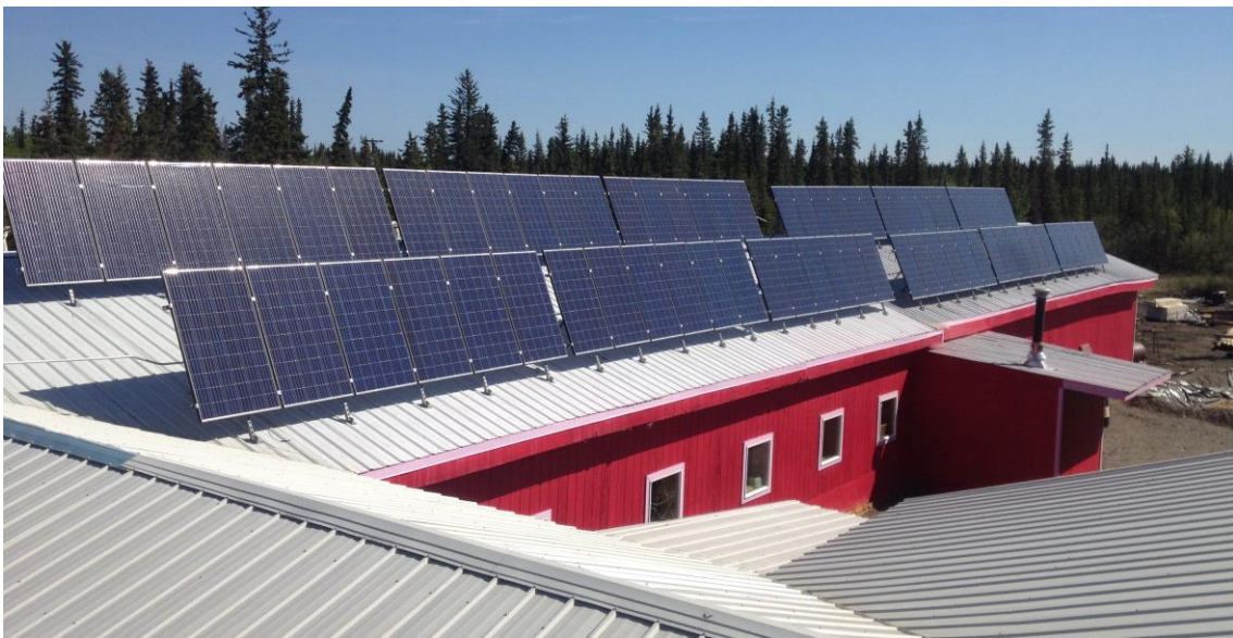
Figure 5. The 18kW Solar PV array installed with 100% local labor on the roof of the Fort Yukon Tribal Hall
