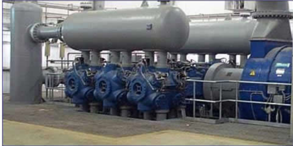
Figure A.1-2 Integral Reciprocating Natural Gas Compressor 68
