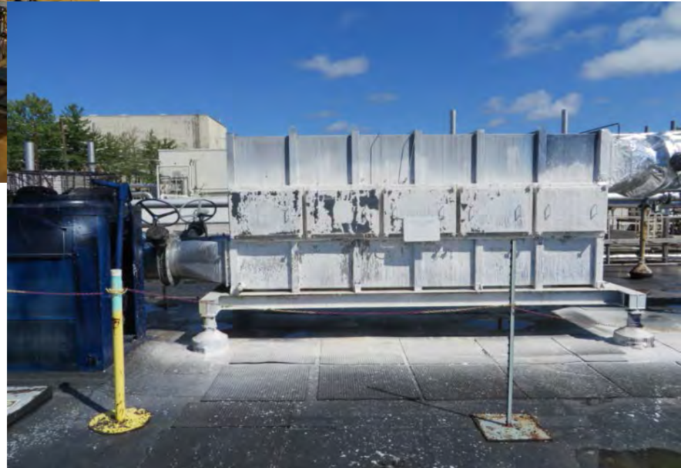
Building 3038 HEPA Filter Housing
