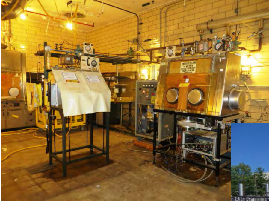
Building 3038 Glove Boxes
