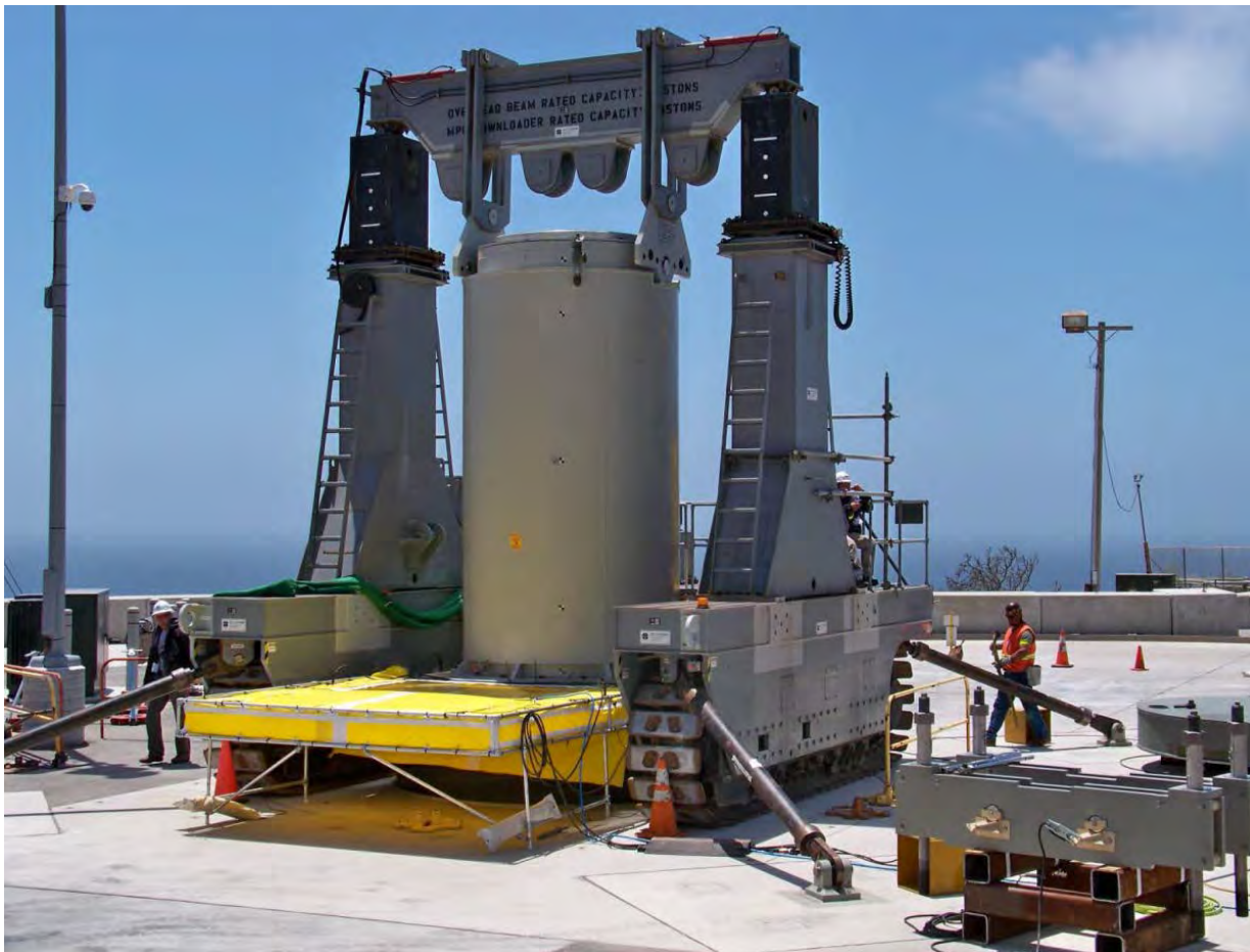
Figure 4-14 Holtec Below Grade Vertical Canister Transfer Facility at the Diablo Canyon ISFSI
