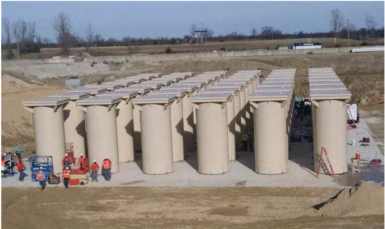
Figure 3-8 Holtec UMAX VVM set on the Base Mat at the Callaway ISFSI
