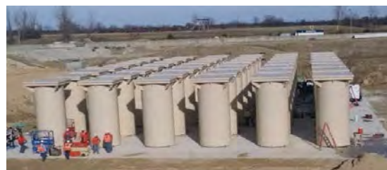
DPCs will be stored underground in the UMAX system at the Callaway ISFSI
