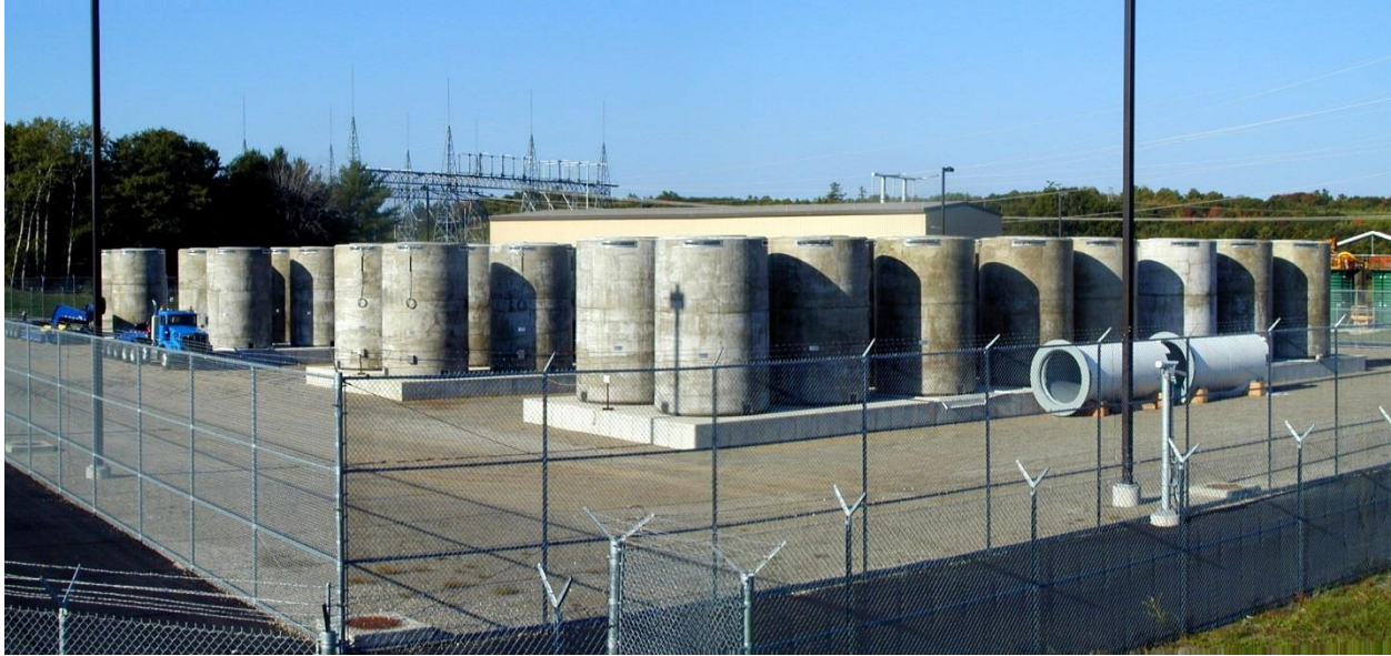
Figure 4-11. An Independent Spent Fuel Storage Installation Facility
