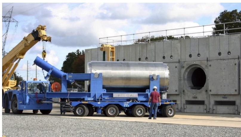
Figure 4-13. Horizontal Concrete Cask Storage
