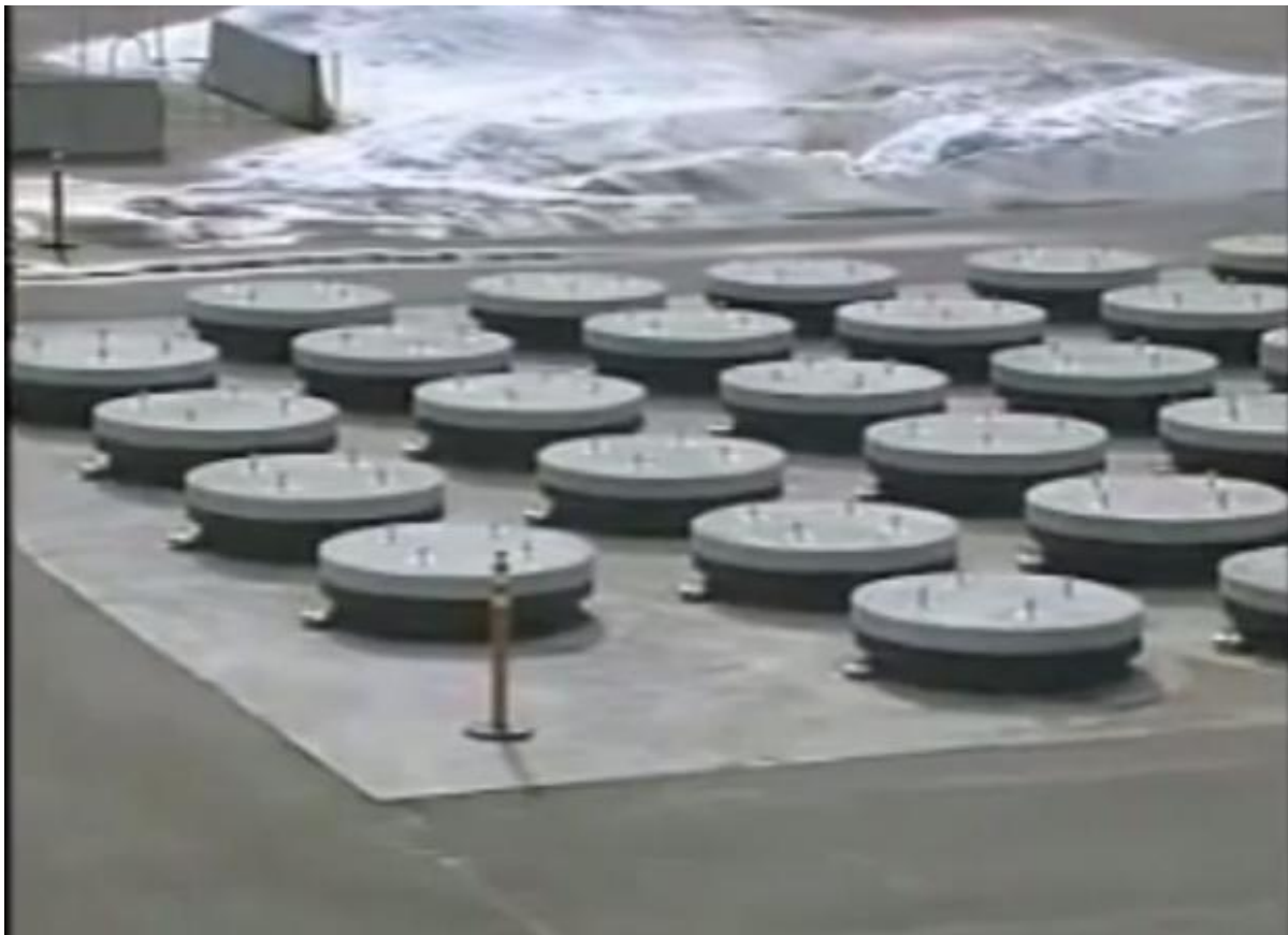
Figure 4-14. In Ground Storage at Bruce Power
