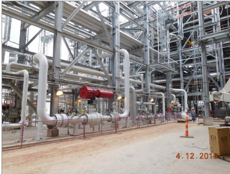
Train 2 - Fuel Gas Area (Turned Over to Start-Up)
