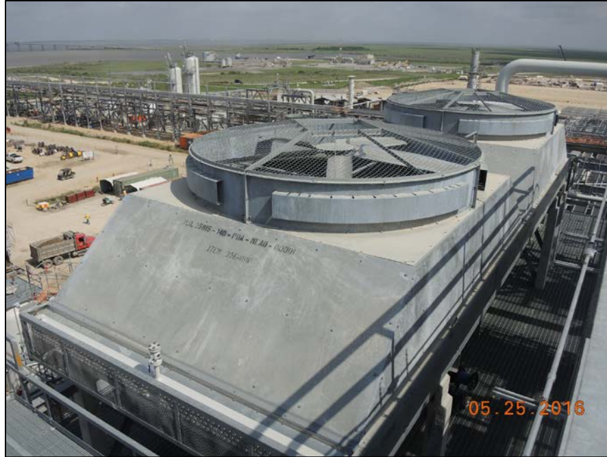
Train 3 - Stabilizer Condenser Air Cooled Exchanger in Utility Pipe Rack
