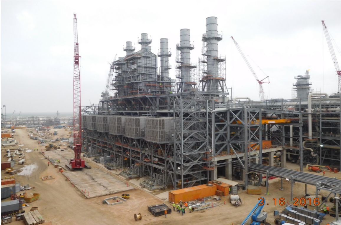
Train 3 – Compressor Area
