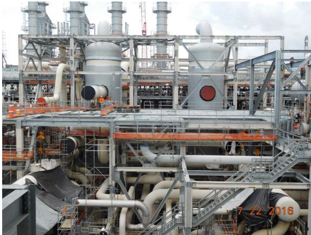
Train 4 – Propane Refrigeration Area
