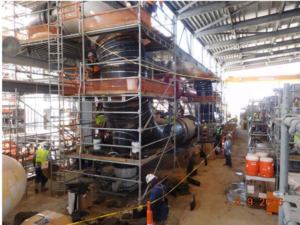
Train 3 – Insulating Pipe above the Compressor Deck
