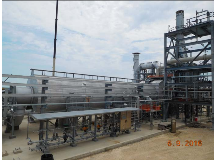
Train 3 - Thermal Oxidizer Area
