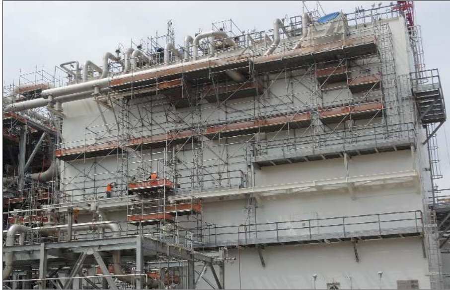
Train 4 - North Side of Methane Cold Box
