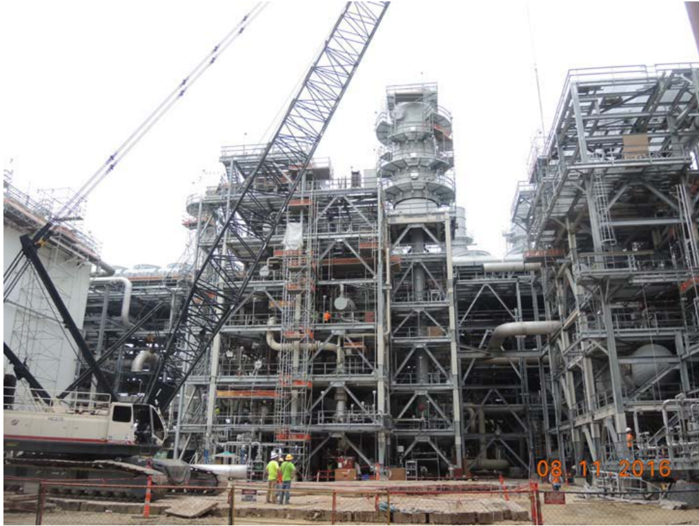
Train 4 – Heavies Removal Area
