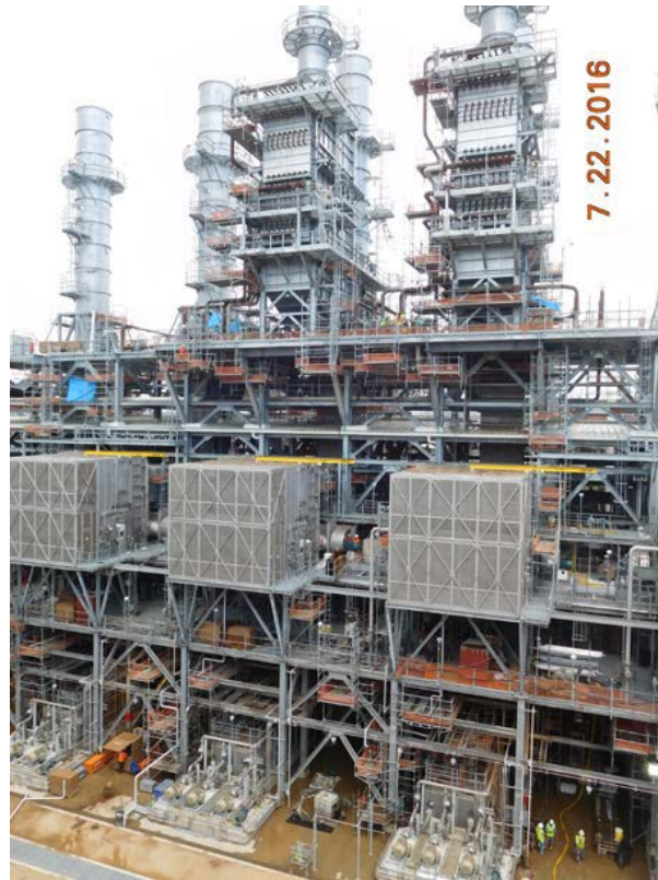
Train 3 – Compressor Area
