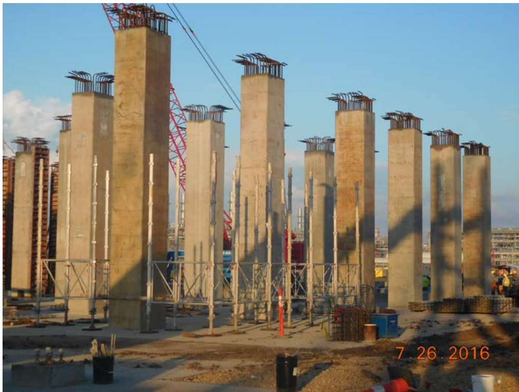
Train 5 – Commenced Installation of Shoring on Northeast Side of Propane Compressor Foundation
