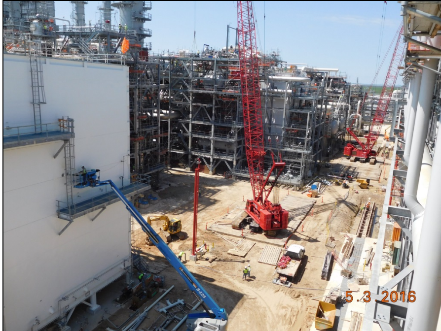
Train 3 - West of ISBL - Methane Cold Box, Heavies Removal Unit and Ethylene Cold Box Areas
