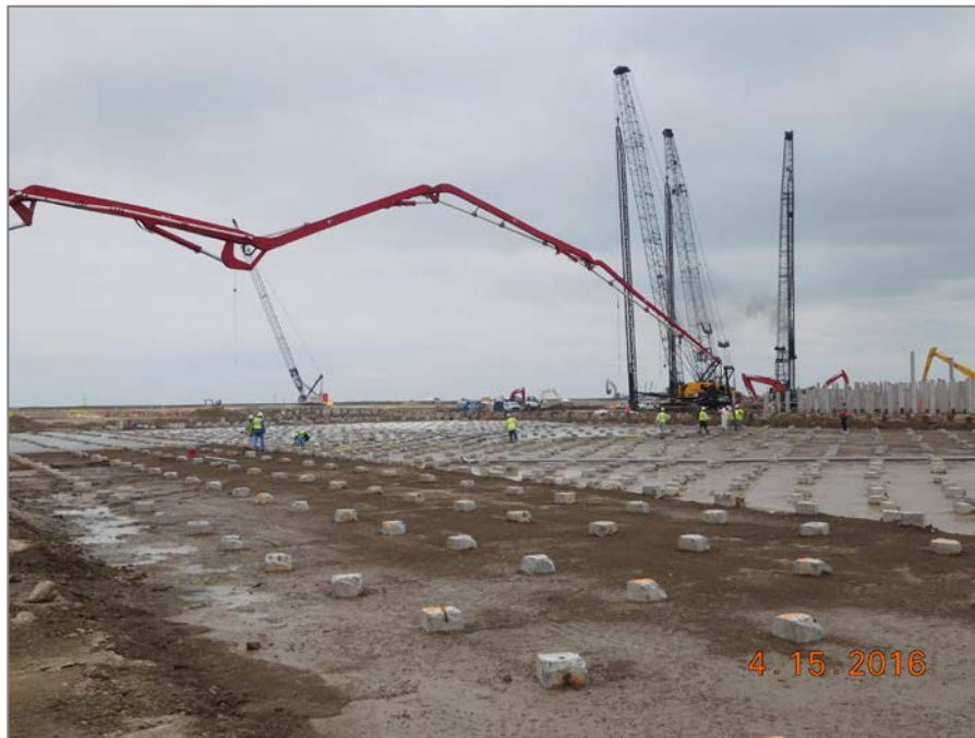
Train 5 - Mudmatting Compressor Area
