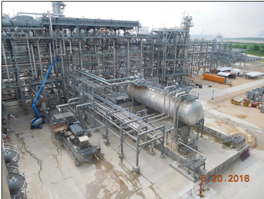
Train 2 - Regeneration Gas Compressor & Hot Oil Area
