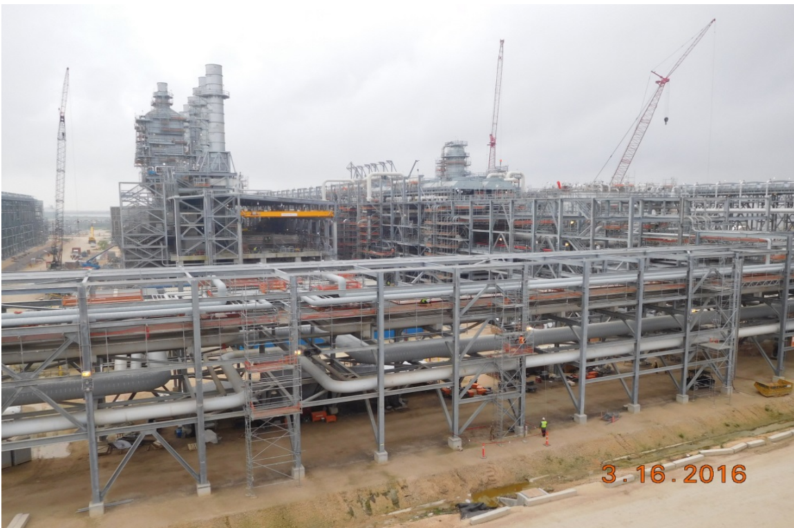
Train 2 – View from North (Common R02 Rack, Compressor Area and Cryo Rack)
