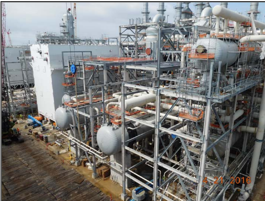
Train 4 - Propane Refrigeration Area
