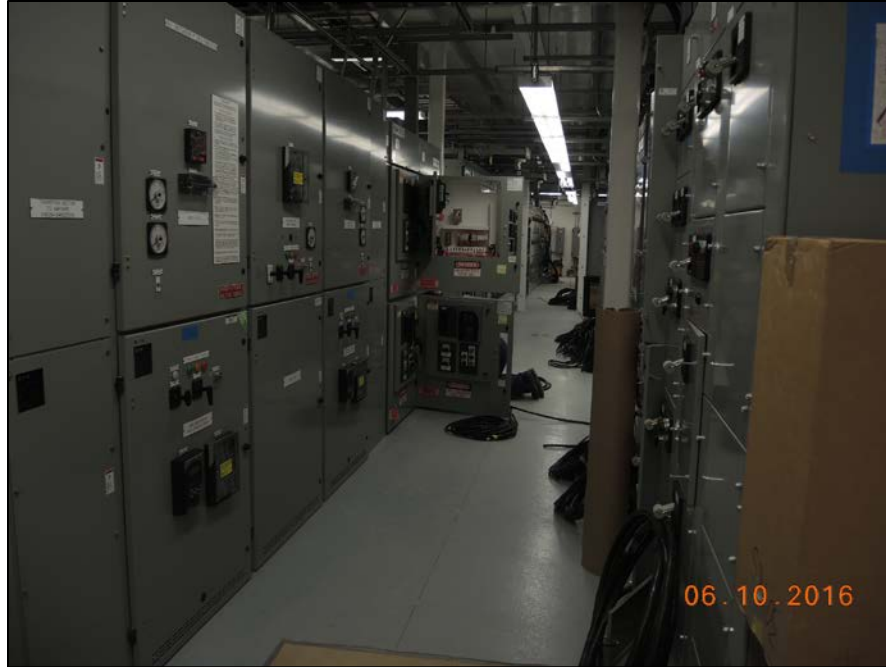
Train 4 - Propane Substation Gears
