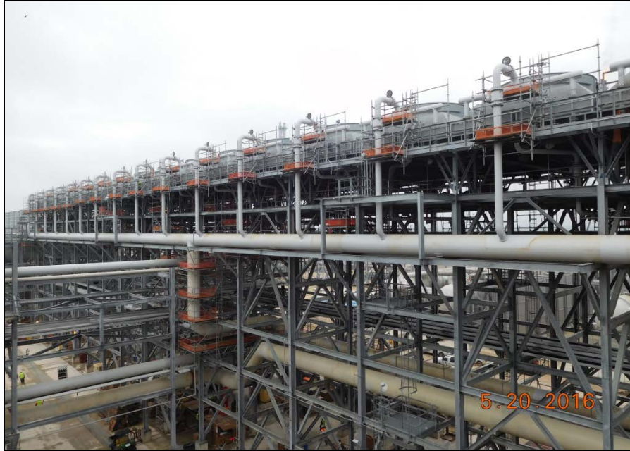
Train 3 - Propane Condenser Area
