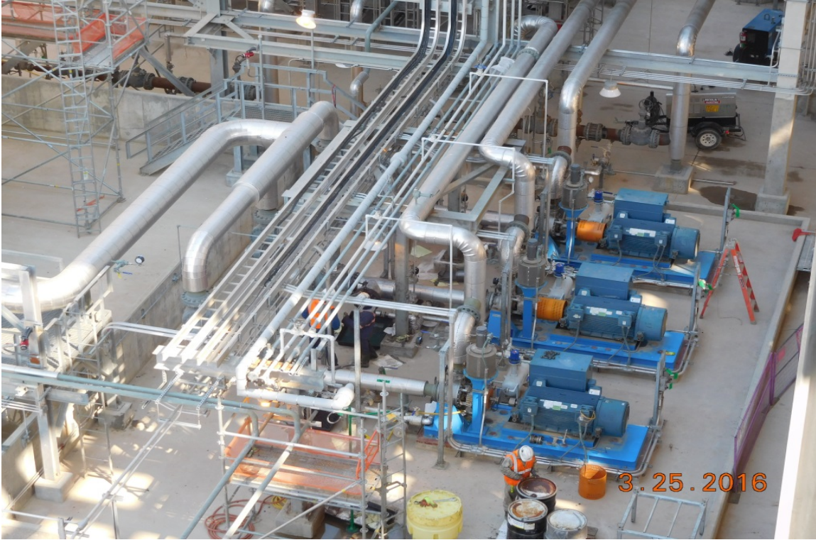
Train 2 – Hot Oil Pumps
