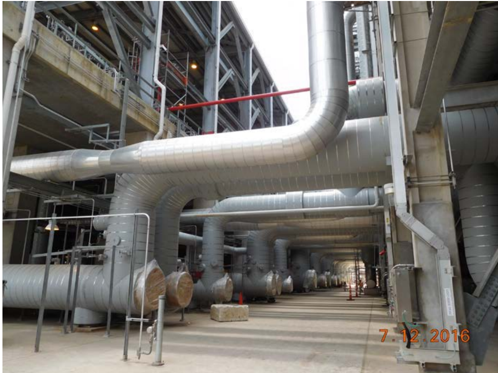
Train 2 – Alleyway between Compressor Area and Cryo Rack
