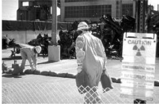
Hazard area secured with fencing and signs
