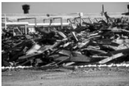
Low-level radioactive scrap metal from a building demolition at uranium processing facility
