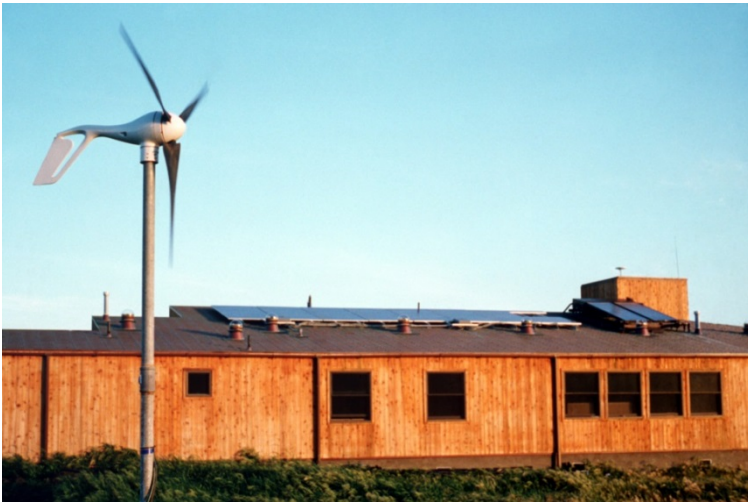
Facility Scale Hybrid System, NPS Range Station, San Miguel Island, CA. Photo by Kent Bullard, NREL 6325496
