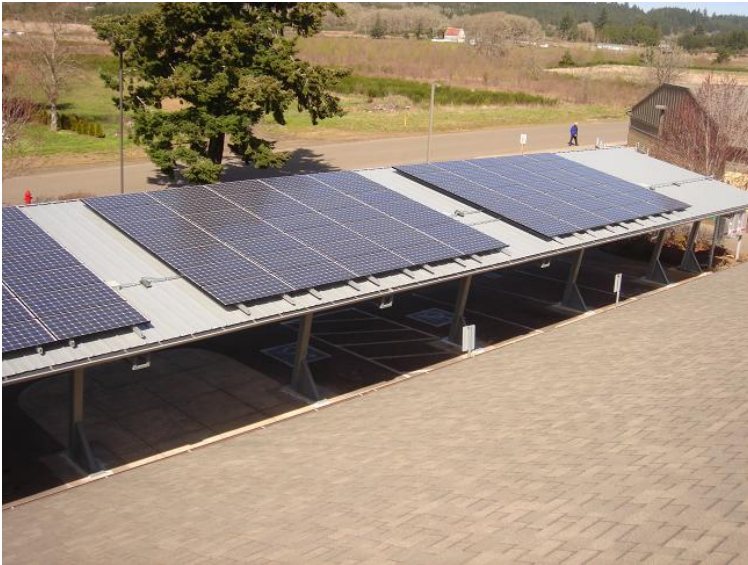
PV Panels on Grand Ronde Tribal Housing Authority carport. Photo by GRTHA, NREL 11659046
