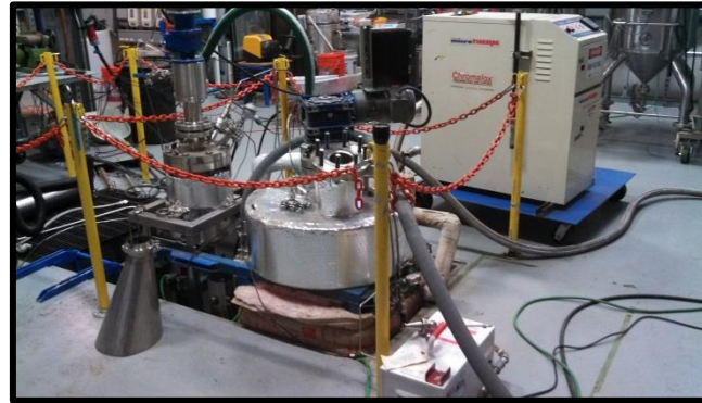
100 Liter Pretreatment Reactor (NEW)
