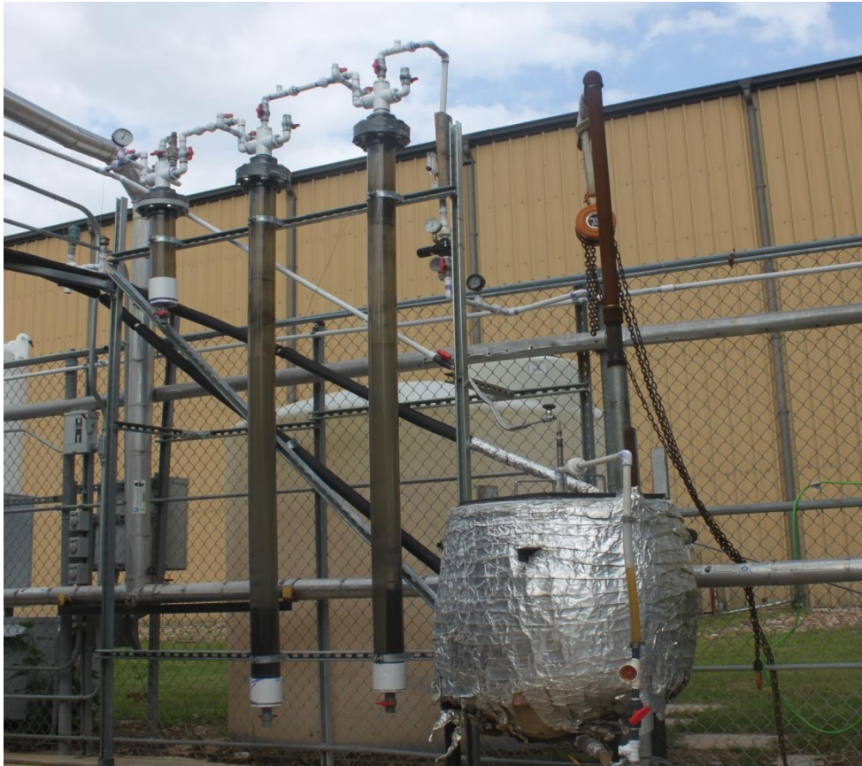
Kettle exterior and CO 2 scrubber columns
