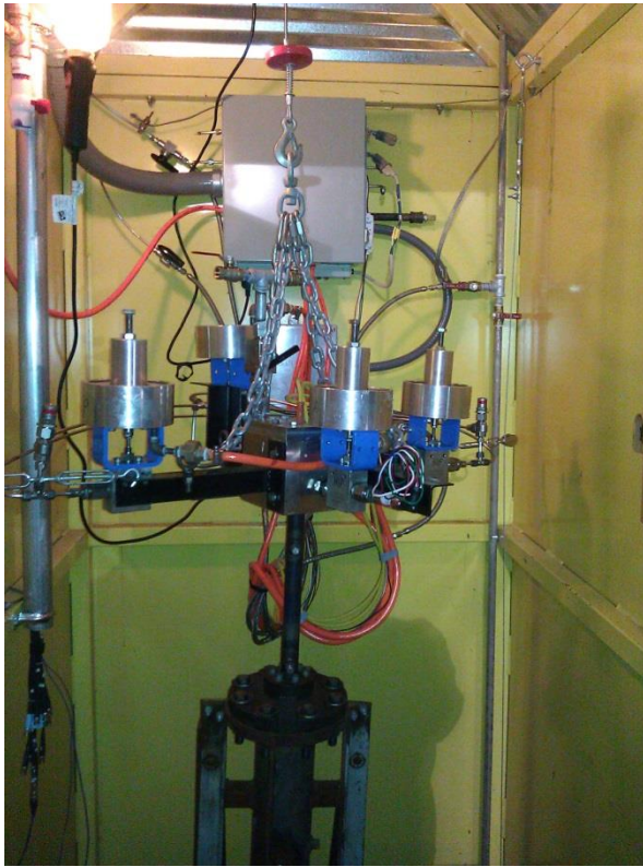
Manifold installed in bunker
