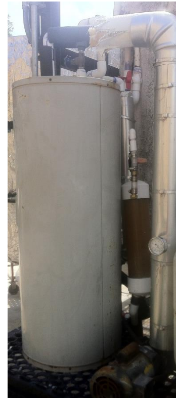
Heater and pump
