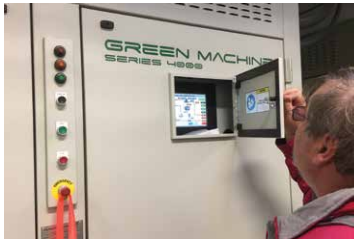
Dan Winters, manager of Unalaska's municipal utility, monitors a generator from recaptured (waste) heat.
