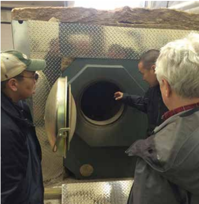
The research team examines a wood boiler system in Kobuk.
