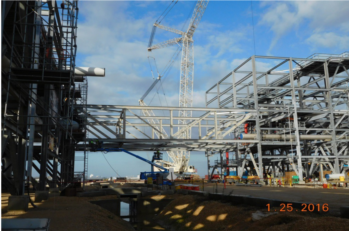
Train 4 – Pipe Bridge to R02 Common Rack
