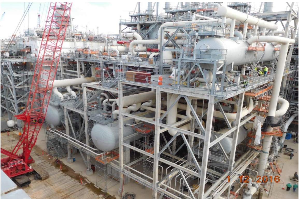
Train 2 – Refrigeration Area Progress
