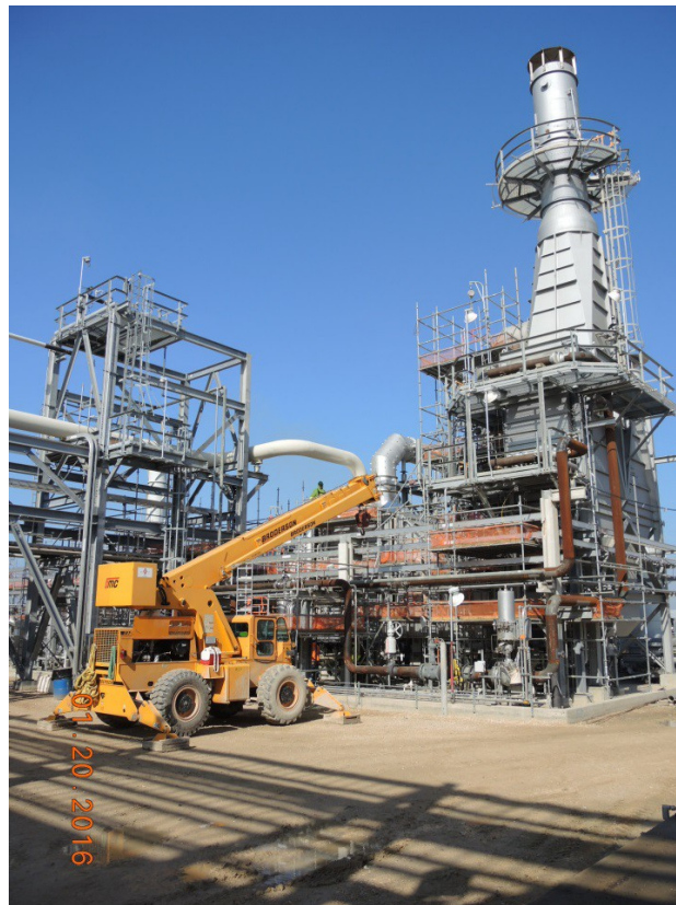
OSBL Train 4 – Hot Oil Waste Heat Recovery Coil in Thermal Oxidizer Area
