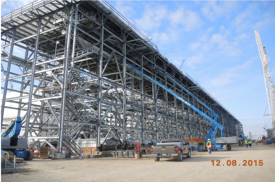
Train 4 – Propane Condenser Area
