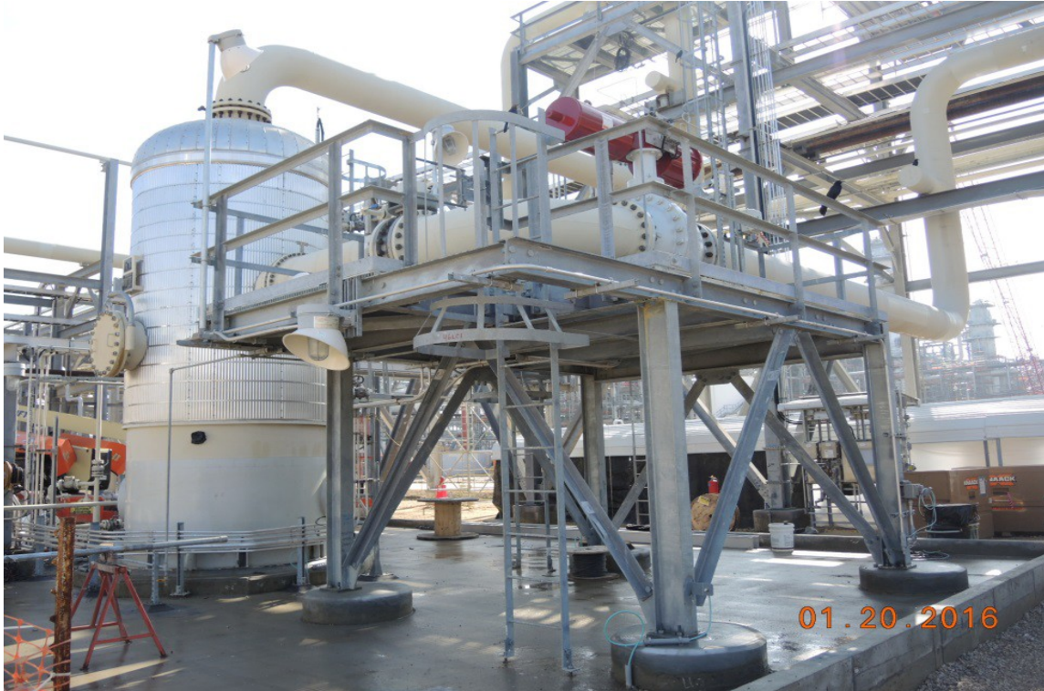
OSBL Train 4 – Hot Oil KO Drum in Thermal Oxidizer Area
