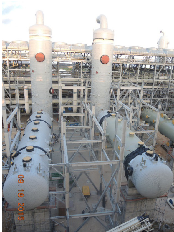
Train 4 – Propane Refrigeration Area
