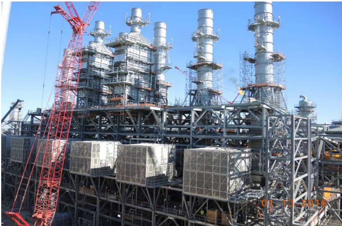
Train 3 – WHRU Compressor Area
