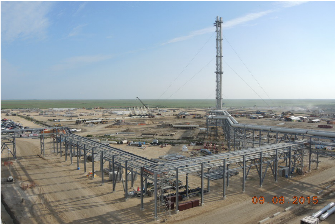
OSBL Piperack Utilities and Flare Stack
