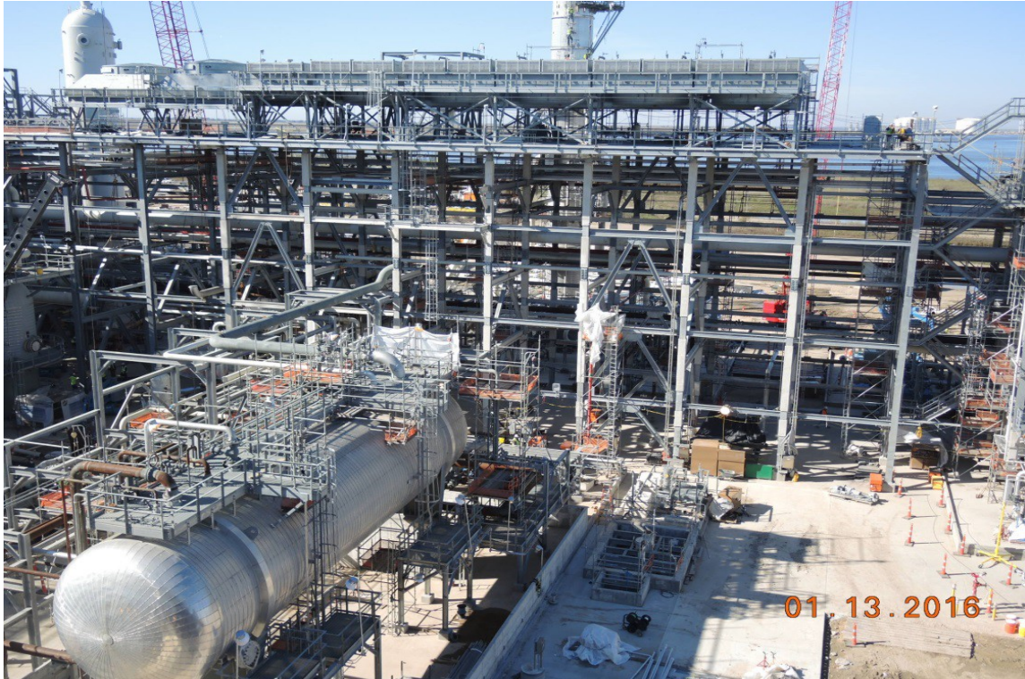
Train 4 – AGRU Air Coolers and Pipe Rack Areas
