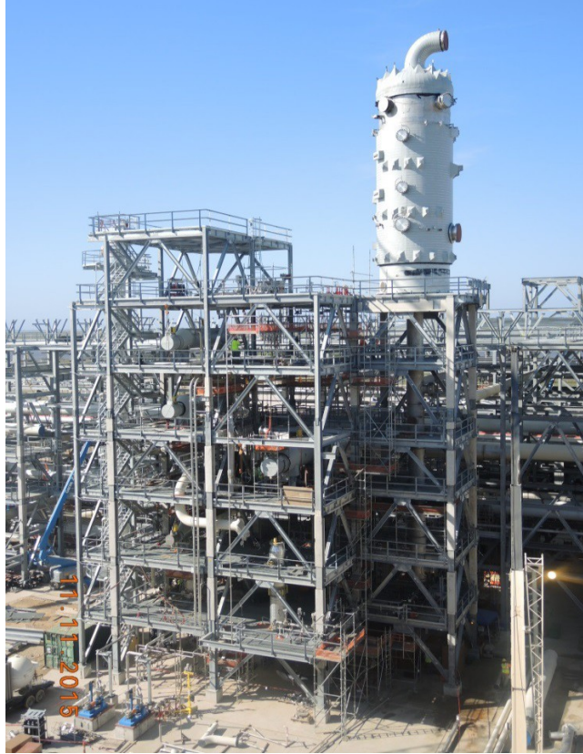
Train 4 – Heavies Removal
