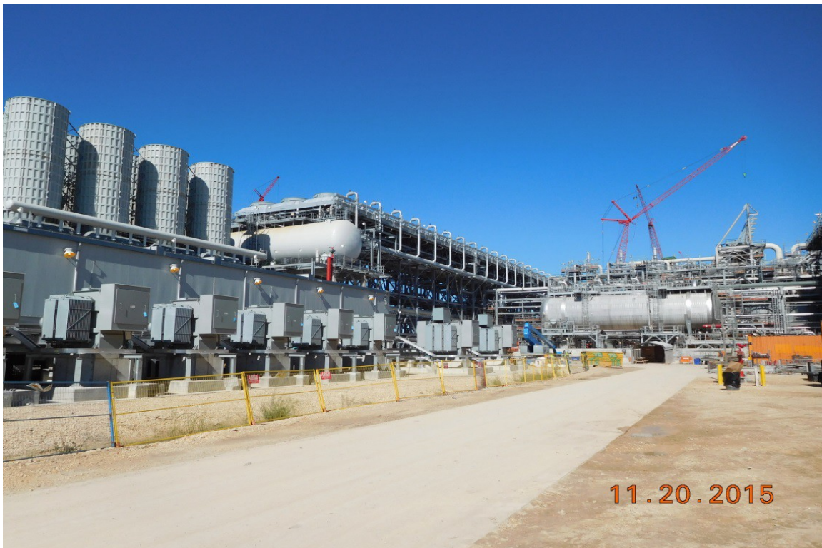
Train 2 – Propane Substation Building
