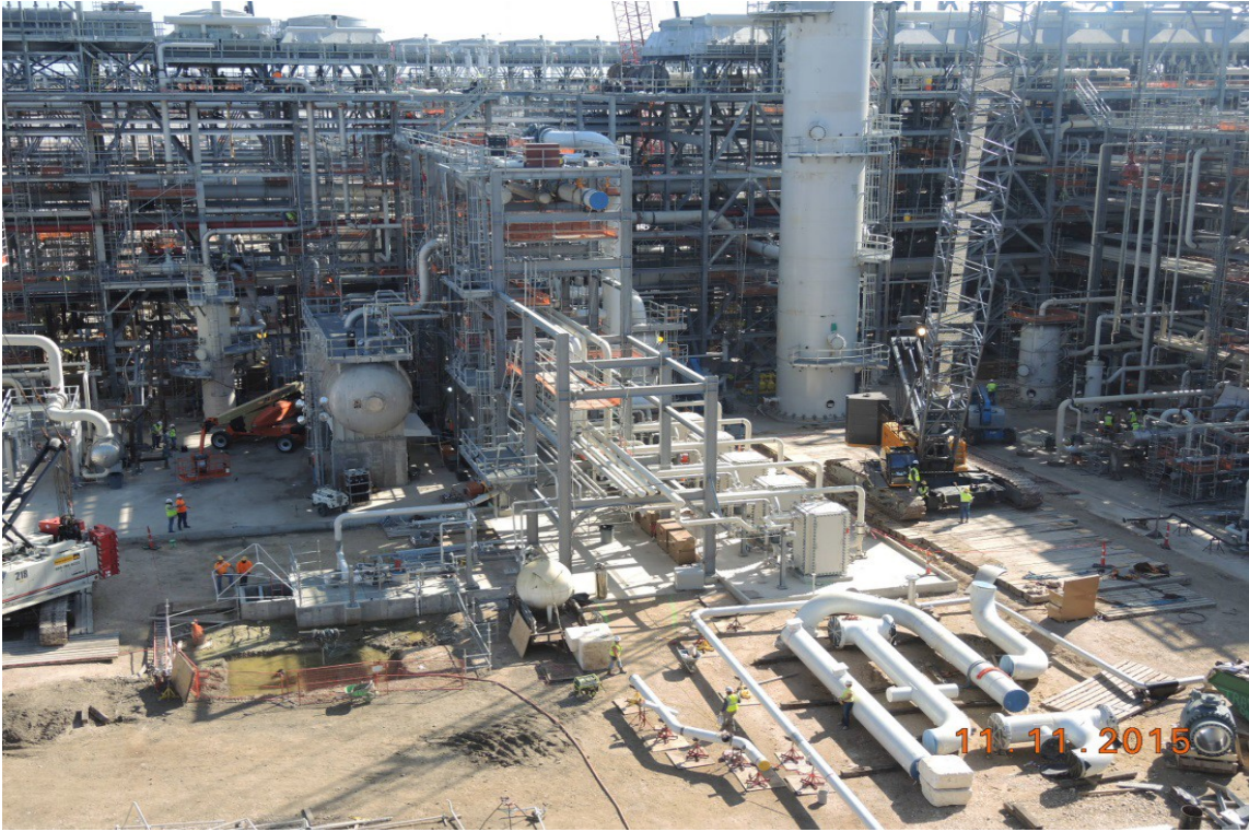
Train 3 – Amine Regen and Acid Gas Removal
