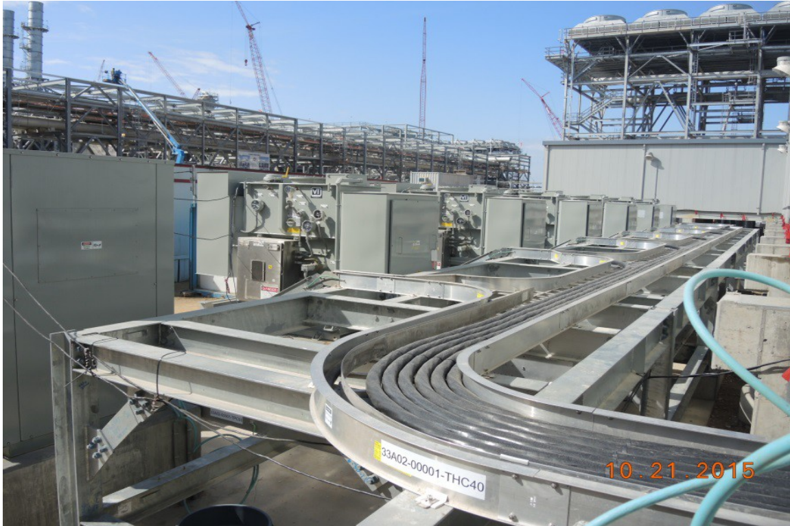
Train 3 – Cable Tray and Cable going into the Compressor Substation
