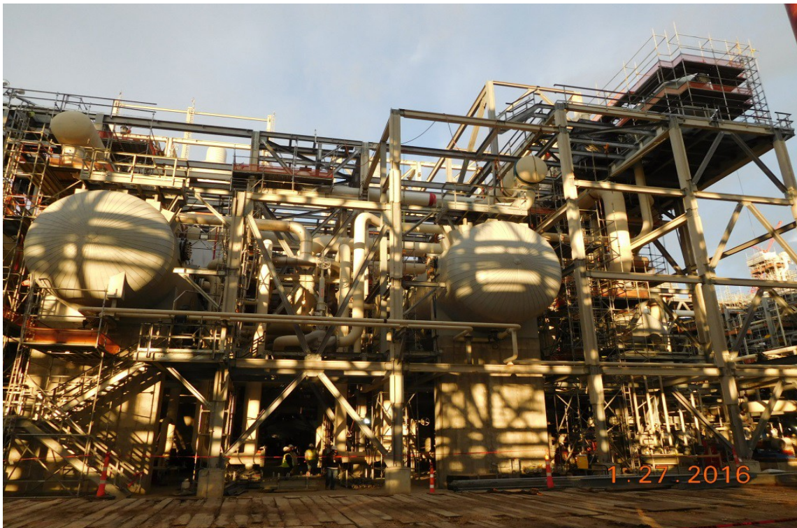
Train 4 – Propane Refrigeration Area
