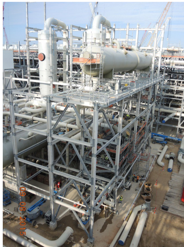
Train 3 – Propane Refrigeration Area
