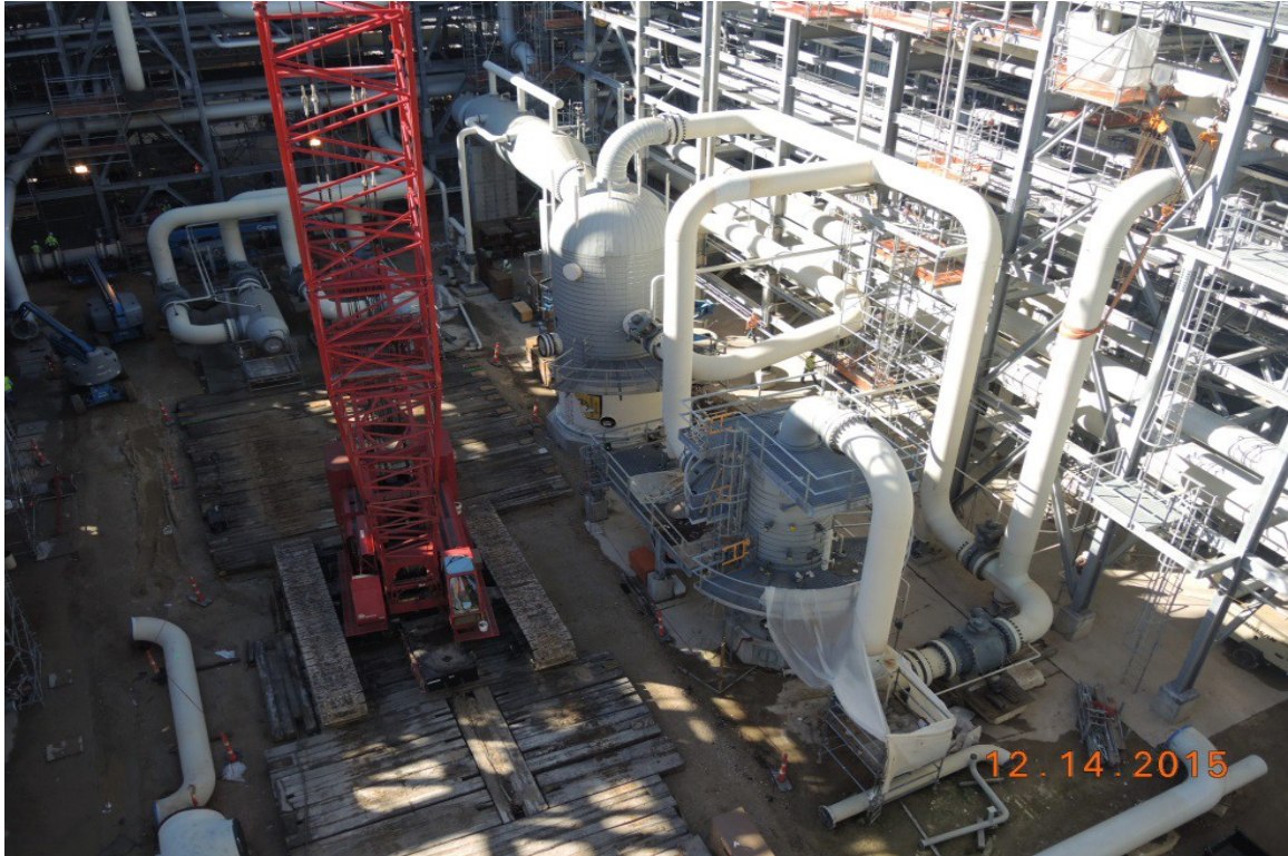
Train 3 – Dryer Feed KO Drum and Dryer Inlet Filter Coalescer
