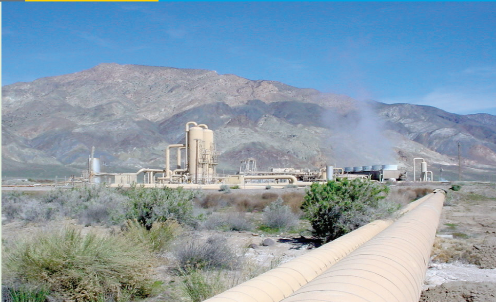
Dixie Valley Bottoming Binary Plant: Terra-Gen was funded by the American Recovery and Reinvestment Act of 2009 to demonstrate the technical and economic feasibility of electricity generation from nonconventional geothermal resources of 223°F, employing the first commercial use of a supercritical cycle at a geothermal power plant inlet temperature of less than 300°F. Since September 2012, the plant has been online and producing 6 MW gross.
