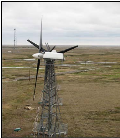
Chaninik Wind Group's Thermal Heating Project (AK)
