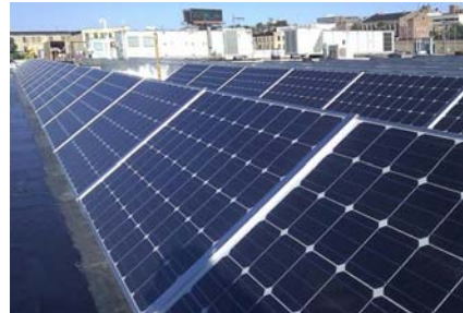
The Forest County Potawatomi Tribe's 30-kW solar PV system on the roof of its administration building in Milwaukee, WI. Photo from the Forest County Potawatomi Tribe, NREL 20107.
