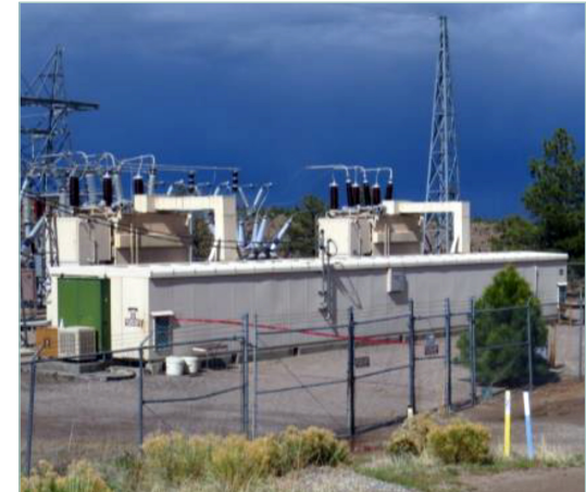
Figure 1-1. The 13.8-kV substation TA-53-0070
