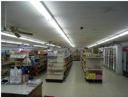
LED lights installed in the Corporate Store
