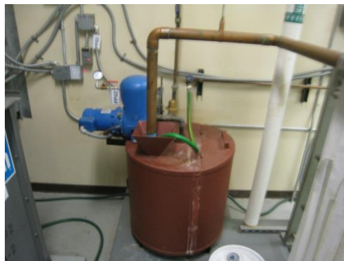
6 gallon Water heater installed in the Store.
