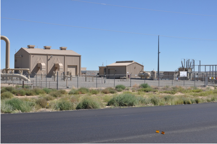
Photograph 1. Bisti Substation from Highway 371, looking east/southeast.
