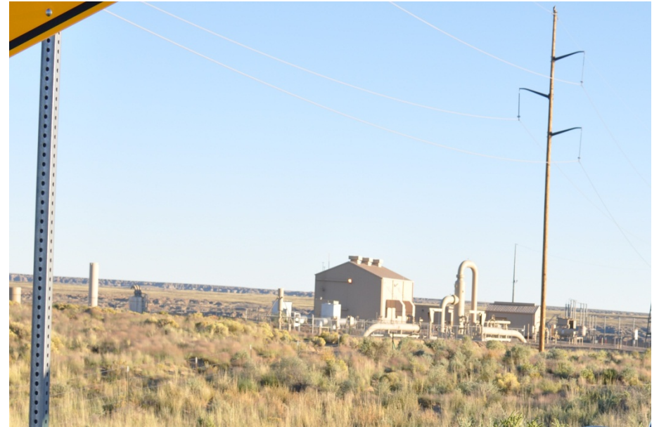
Photograph 39. View of the Natural Gas Compressor Station from area between the Bisti Substation and the Compressor Station along Highway 371, looking south/southeast.
