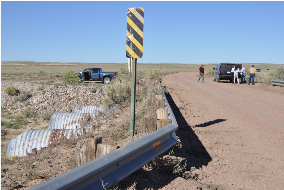
Photograph 22. View of culvert along County Road 7500 where County Road crosses eastern portion of Site 2 that extends in a southerly direction.
