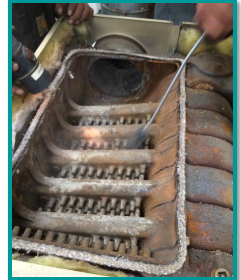
AFTER: Clean flue passage
