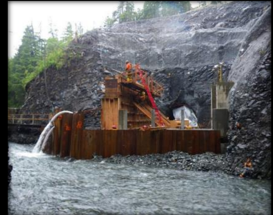
Humpback Creek Hydroelectric Cordova, Alaska
