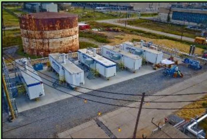
New natural gas package boilers.
