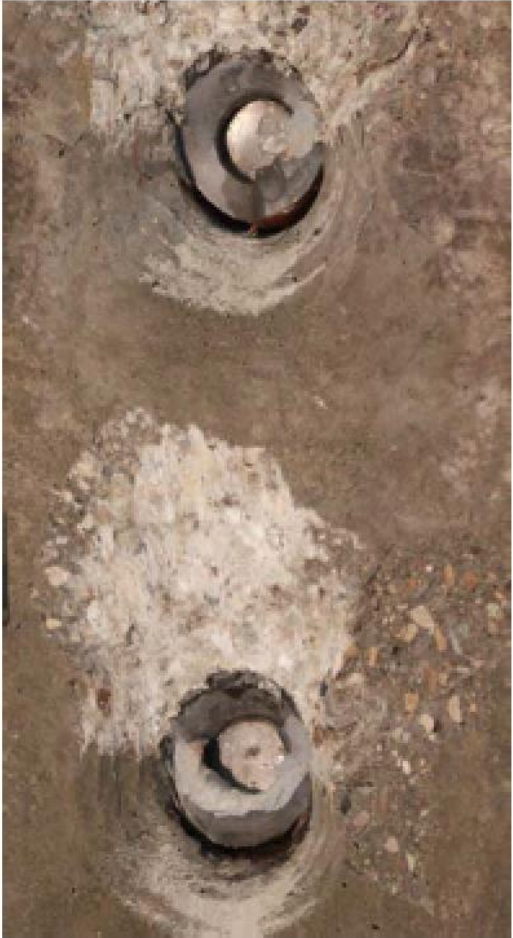
(b) Fractured Couplers and #11 Anchor Rebars in Specimen Block
