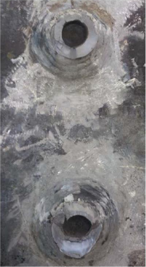
(c) Fractured Couplers Welded at Basement
