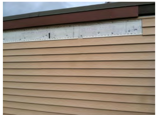
Figure 102. Missing vinyl siding on exterior wall.
