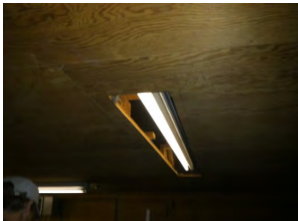
Figure 31. Shop ceiling showing recessed lighting in unsealed ceiling penetration.
