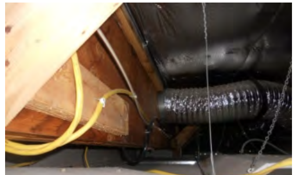
Figure 60. Existing ceiling insulation and duct work penetrating structural roof member.
