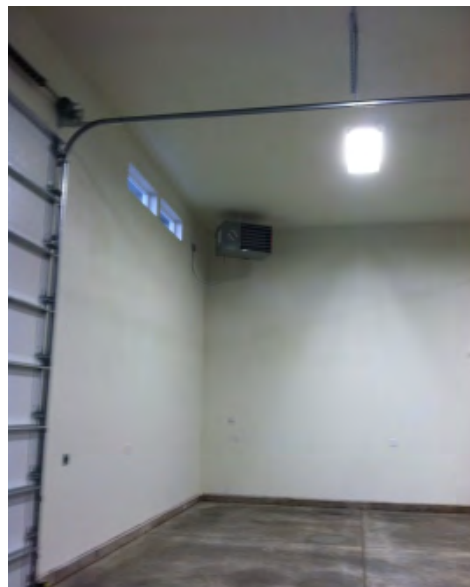
Figure 36. New Shop interior showing Modine unit heater and high output T-5 linear fluorescent lighting.
