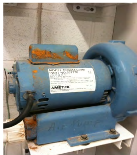
Figure 118. Spa air pump with significant corrosion.
