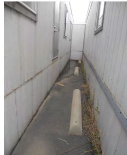
Figure 12. Standing water in contact with building siding in rear alcove.
