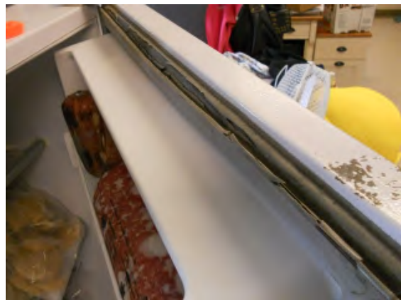
Figure 24. Compromised door gasket on Signature2000 freezer unit
