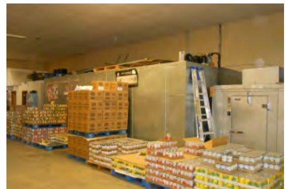
Figure 19. Food Distribution Warehouse freezer and cooler units
