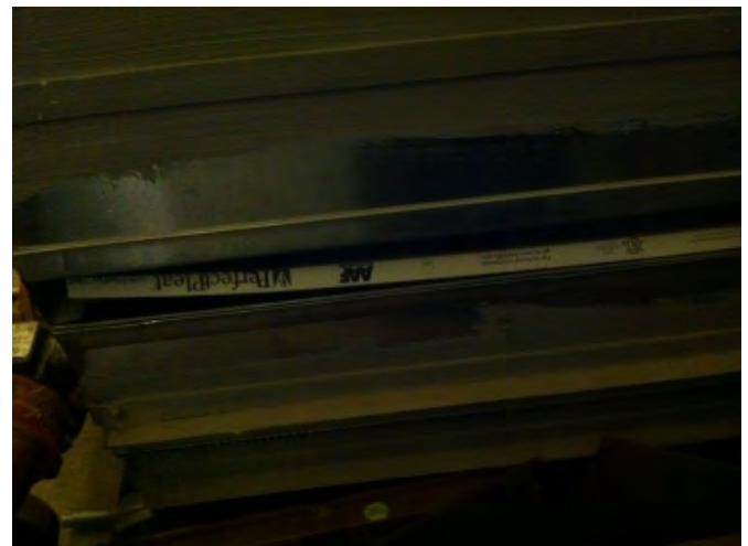
Figure 84. HVAC air handler with missing filter door
