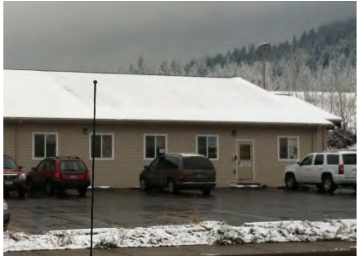
Figure 43. Felix Aripa roof detailing differences in snow melt over connected sections of the roof. Note color of roof deck on north side of structure.
