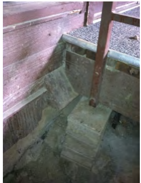
Figure 57. Outside air intake beneath front entry walkway too close to grade level in very dark and moist location
