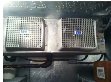
Figure 91. Condensation dripping from ceiling in walk-in freezer.
