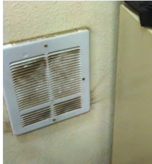
Figure 32. Example electric wall heater with dust and debris noted.
