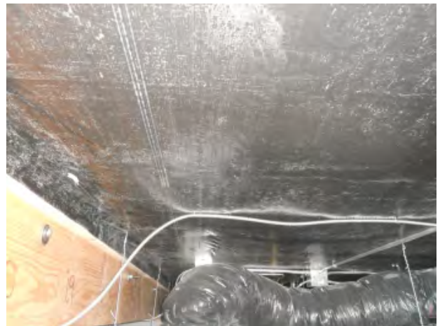
Figure 9. BIA attic detailing rigid insulation and flexible ducting
