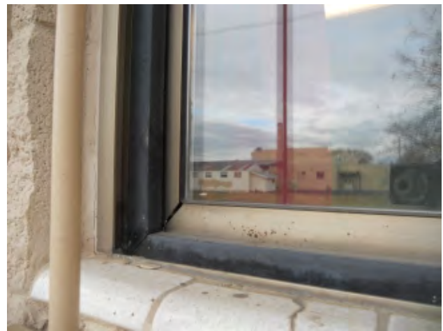
Figure 7. Large gap in poorly fitted window frame.
