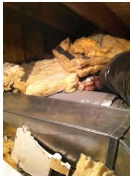
Figure 81. Displaced attic insulation and damaged HVAC distribution system.
