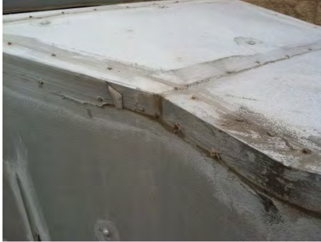
Figure 116. Dectron duct system in need of air sealing
