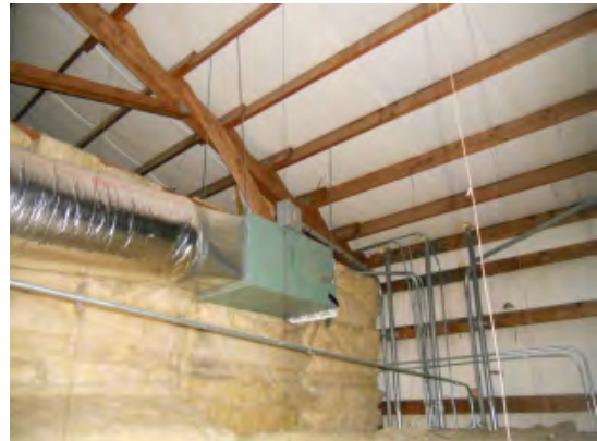
Figure 18. Electric resistance heater unit suspended from roof truss. Note edge of excessively large media filter.
