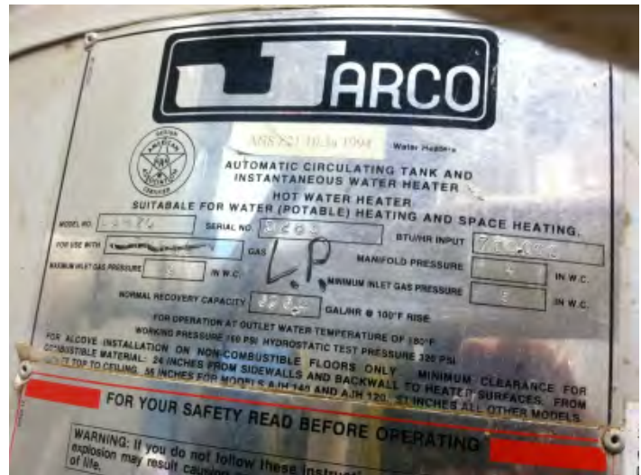
Figure 90. Boiler nameplate specifies natural gas – unknown whether legitimately retrofitted for propane fuel
