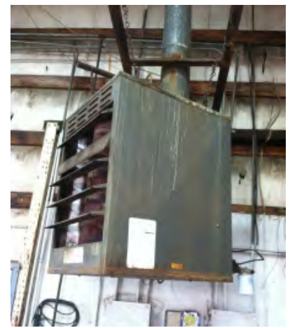
Figure 95. Unit heater with visible corrosion on flue piping and burners.
