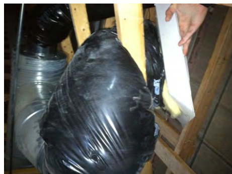
Figure 88. Furnace #F11 disconnected duct blowing into attic
