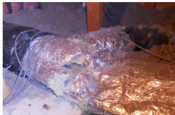
Figure 2. Public Works attic space showing crushed ducting, impacted duct insulation and loose-fill cellulose attic insulation.
