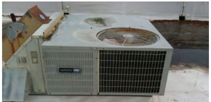
Figure 97. Carrier packaged air conditioner/electric furnace.
