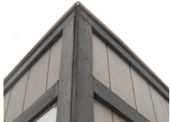
Figure 10. Education building aluminum channel and water impacted cornice.
