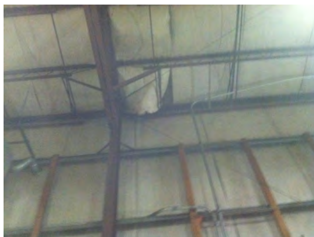
Figure 100. Damaged ceiling insulation noted on interior of structure.
