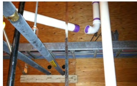
Figure 87. Furnace #F15 combustion air intake line disconnected
