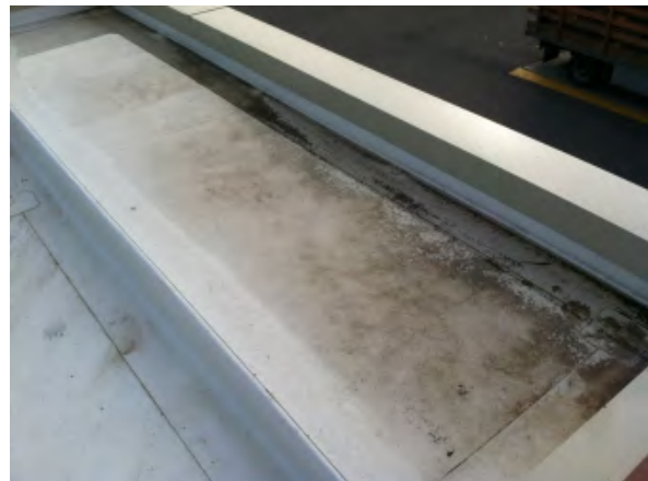
Figure 70. Standing water on roof above entry way.
