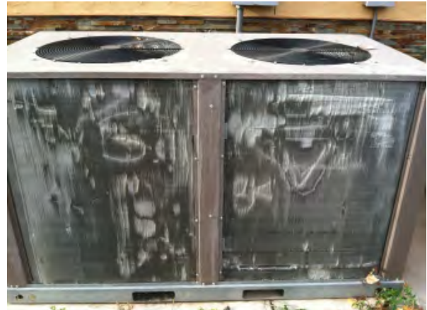
Figure 28. York, 2-ton heat pump detailing extensive damage to the heat exchanger fins.
