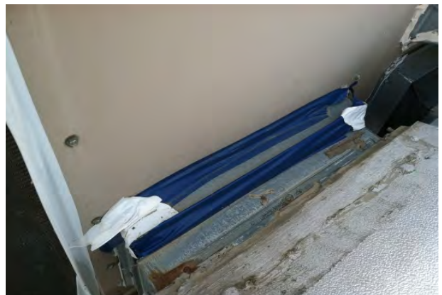
Figure 113. Older York heat pump with compromised duct seals.
