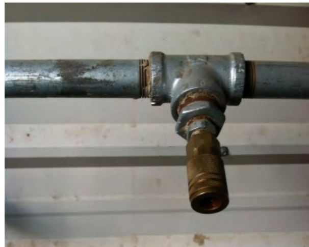
Figure 33. Compressed air distribution system showing significant corrosion around fitting.
