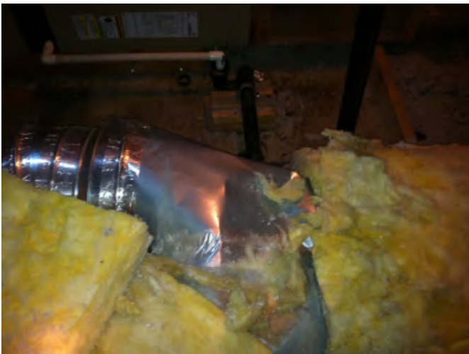
Figure 40. Crushed ducting, impacted duct insulation and foil take on HVAC distribution system.
