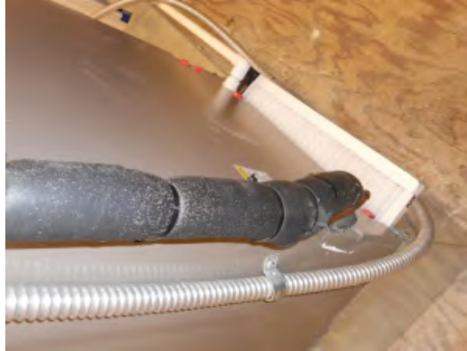
Figure 22. Phase I downstairs AHU with poorly fitted filter and missing filter cover.
