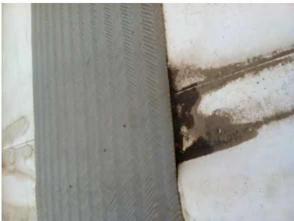
Figure 69. Rubber pathway holding water against membrane roofing seams.
