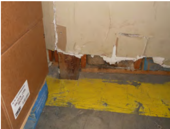
Figure 16. Impacted wall system with visible penetrations to the outside
