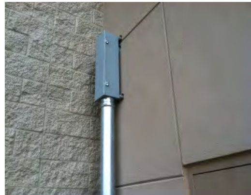
Figure 110. Exterior wall penetration with very poor seal.
