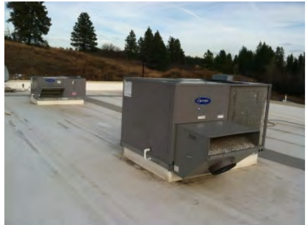
Figure 71. Packaged roof top heat pumps (RTUs).
