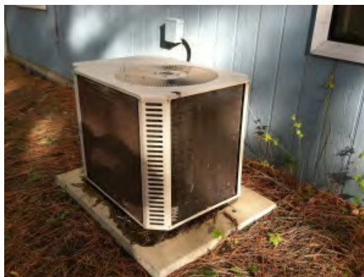
Figure 53. York air conditioner condenser with obvious signs of deterioration.
