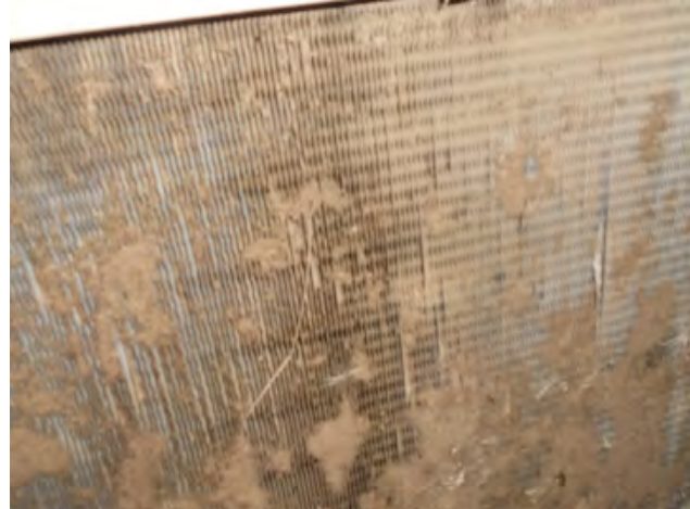
Figure 64. Walk-in cooler condenser fins impacted by debris.
