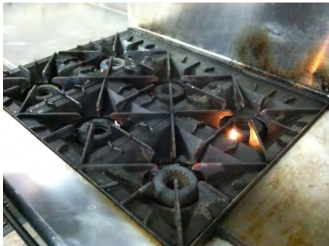
Figure 29. “Lazy” pilot flame observed on commercial range.
