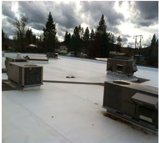
Figure 112. Packaged Heat Pump RTUs.
