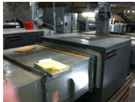
Figure 89. East wing mechanical room.
