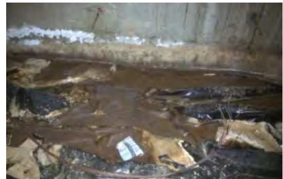
Figure 56. Standing water observed in crawlspace
