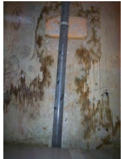
Figure 41. Moisture staining observed on mechanical catwalk adjacent to air handler.
