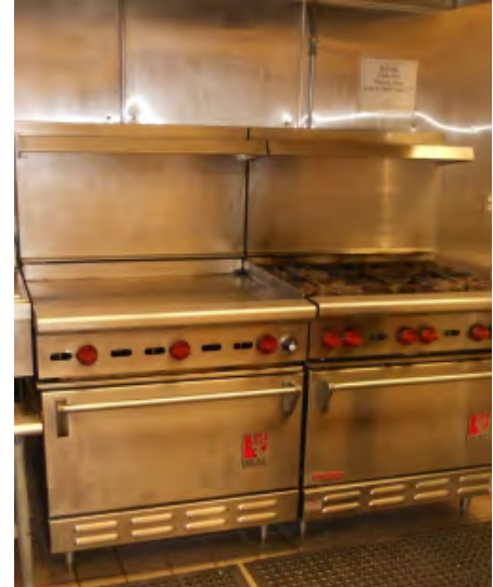
Figure 26. Wolf commercial ovens in kitchen at longhouse.
