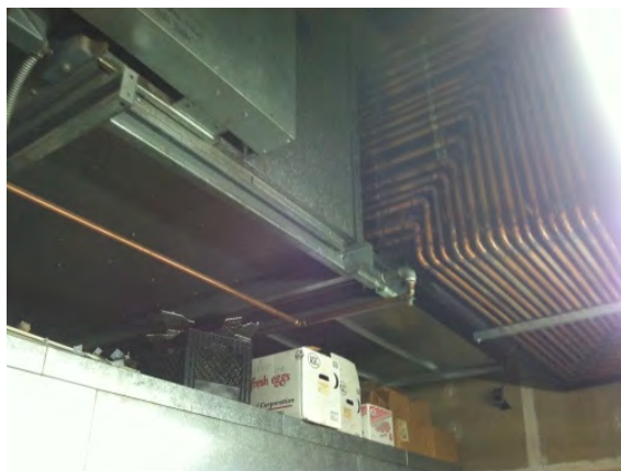
Figure 103. Refrigeration heat recovery system serving building HVAC.
