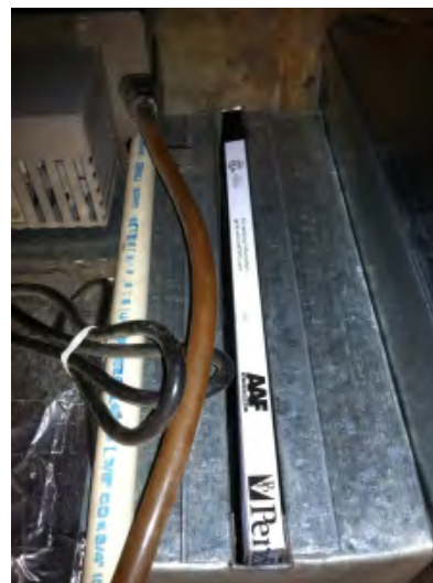
Figure 52. Improperly sized furnace filter with no filter access door in place.
