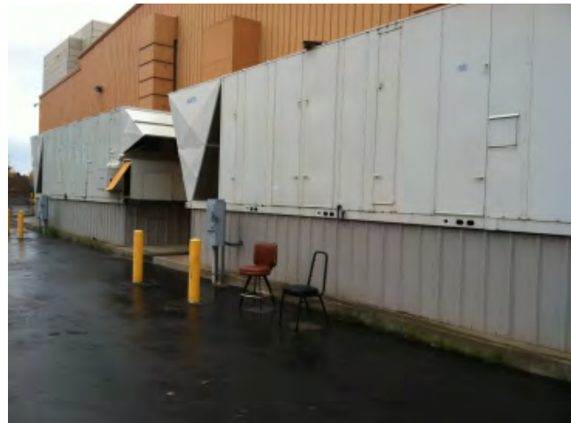
Figure 77. Large, ground mounted, Aaon packaged chillers and propane furnaces.
