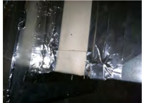
Figure 58. Aluminum duct tape holding together return side of Ruud air handler ducts
