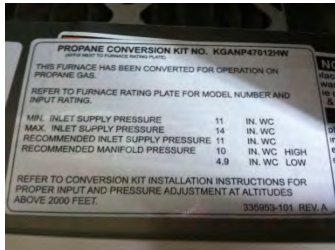
Figure 74. Natural gas to propane conversion label.
