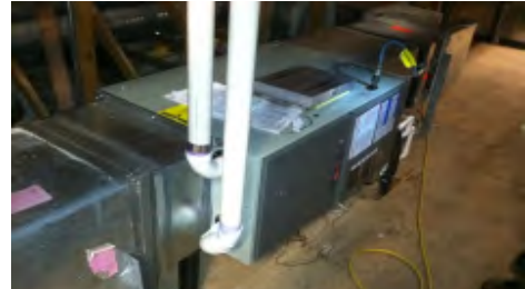
Figure 86. Trane propane furnace/air handlers serving classrooms.
