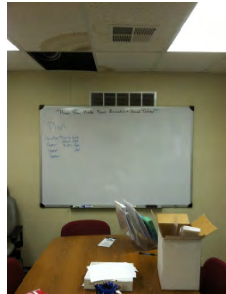
Figure 5. Whiteboard shown blocking the return air register in the Career Renewal office conference room. Also note staining in acoustic tile ceiling from previous moisture intrusion.
