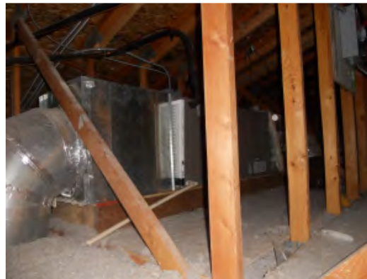
Figure 23. Phase II upstairs AHU with poorly fitted filter and missing filter cover
