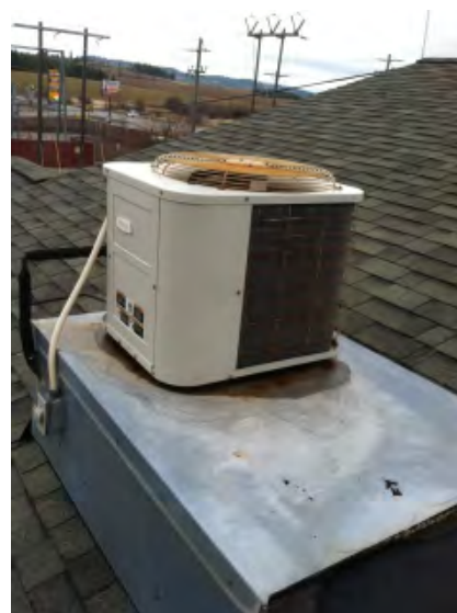
Figure 47. Bryant air conditioner condenser with obvious signs of corrosion and deterioration.
