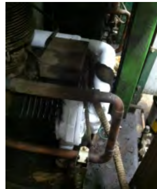
Figure 105. Typical icing observed on refrigeration compressors.
