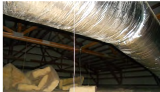
Figure 17. Displaced insulation above suspended ceiling
