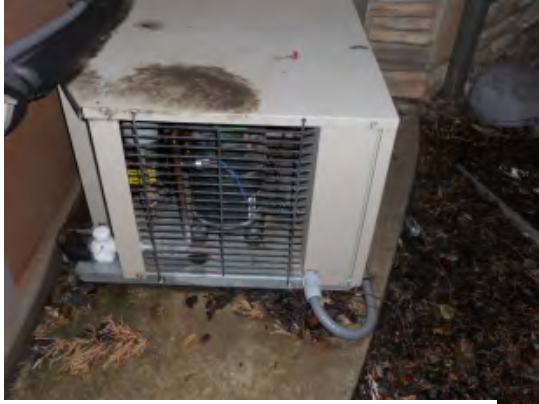
Figure 65. Walk-in cooler condenser with frozen expansion valve
