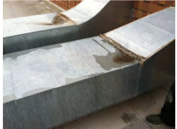
Figure 78. Impacted duct seals on Lennox that serves Presidential Suites.
