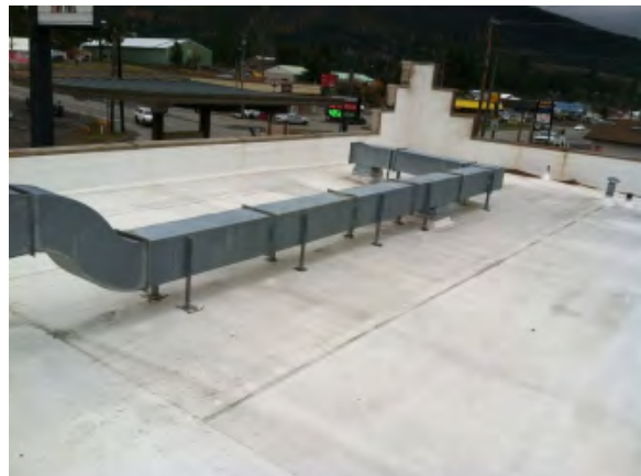
Figure 98. Rooftop HVAC ducting.
