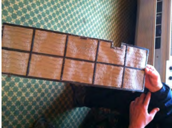
Figure 79. Soiled room PTHP filter in need of maintenance
