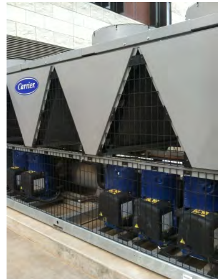
Figure 108. New BMC Chiller
