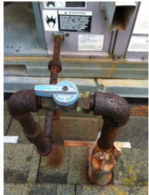
Figure 46. Corrosion noted in propane supply piping.
