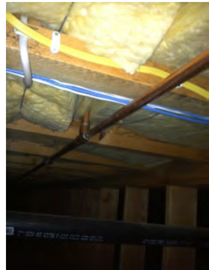
Figure 44. Uninsulated, copper hot water piping in crawlspace
